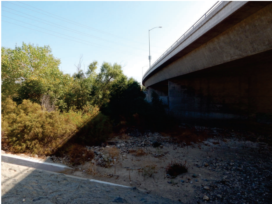
View of the pier walls and cottonwood-willow riparian forest on the east side of the Yorba Linda Boulevard bridge, looking south. The proposed project will require lengthening of the pier walls. November 7, 2019.
