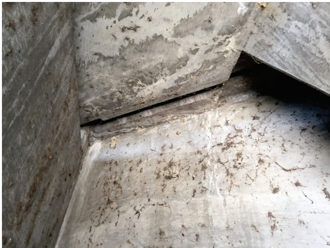
Representative view of crevices with potential bat roosting habitat that were observed at the north abutment of the Yorba Linda Boulevard Bridge.
