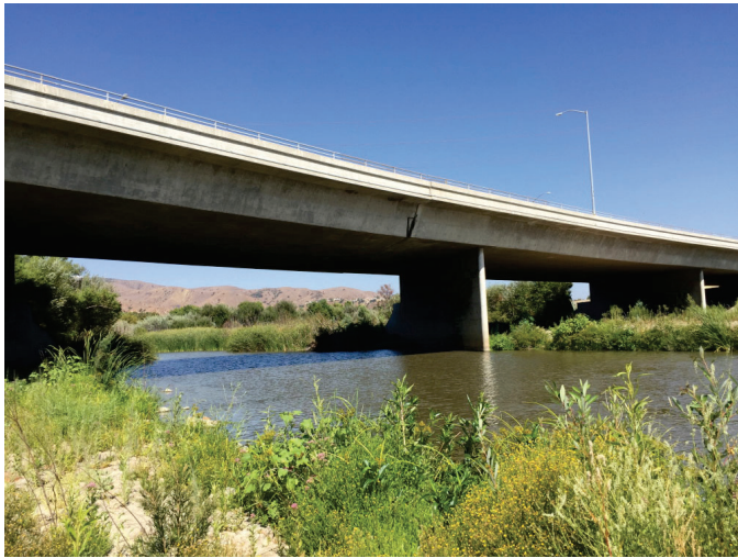
View looking east at the Yorba Linda Boulevard bridge over the Santa Ana River and the surrounding environment. The hinge containing bat roosting habitat suitable for maternity roosting is visible near the middle of the frame.
