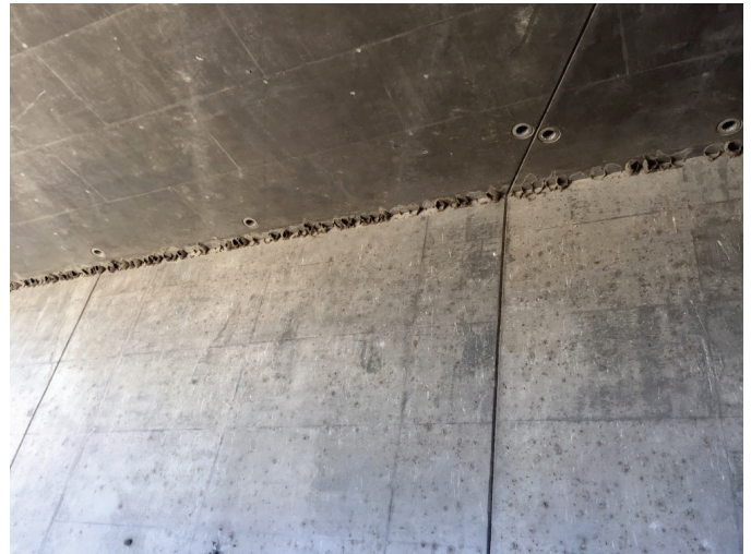
Representative view of cliff swallow nests and weep holes found at the Yorba Linda Boulevard Bridge. Both of these features provide suitable bat roosting habitat.
