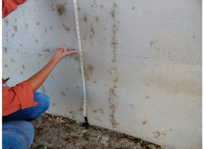
Water marks on the pier wall, showing the ordinary high-water mark. November 7, 2019.
