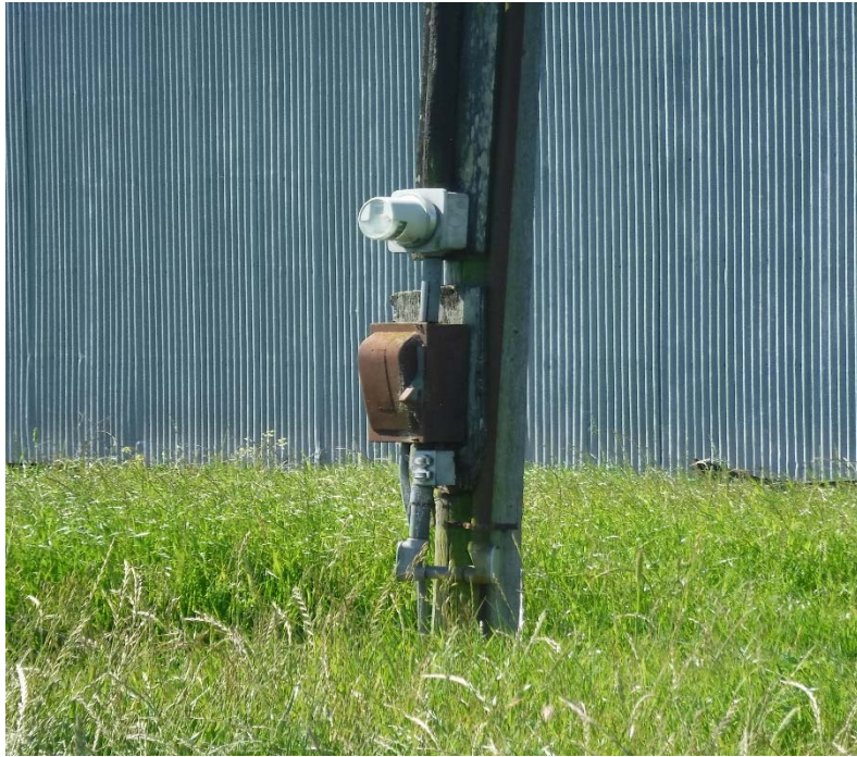
Photo 11: Electrical meter located northeast of the shop building.
