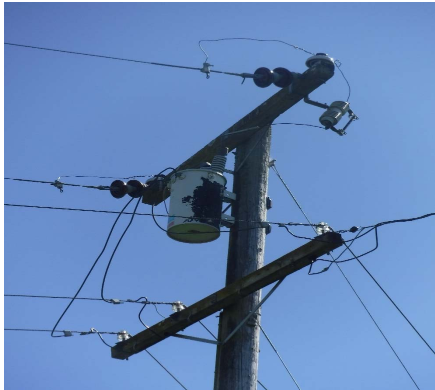
Photo 10: Transformer along the northeast property line of the Subject Property.
