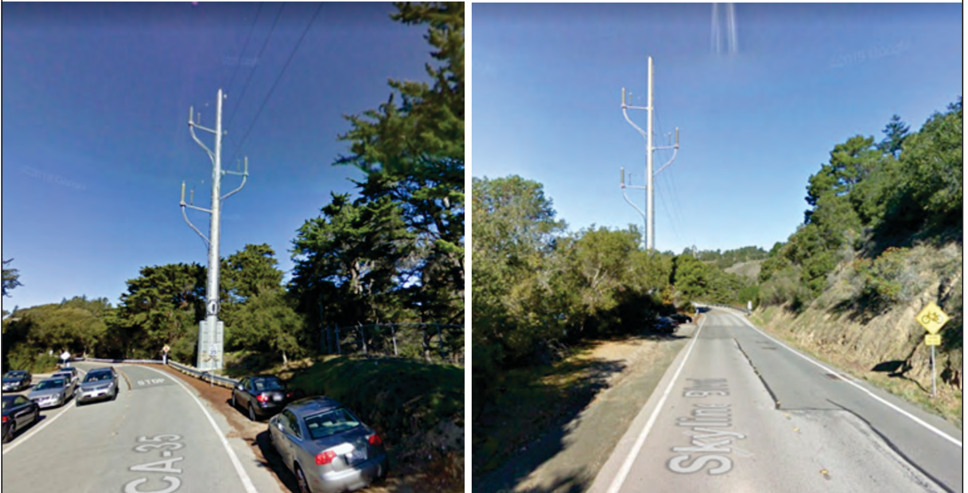
These poles allow the transition of conductors from underground to overhead.
