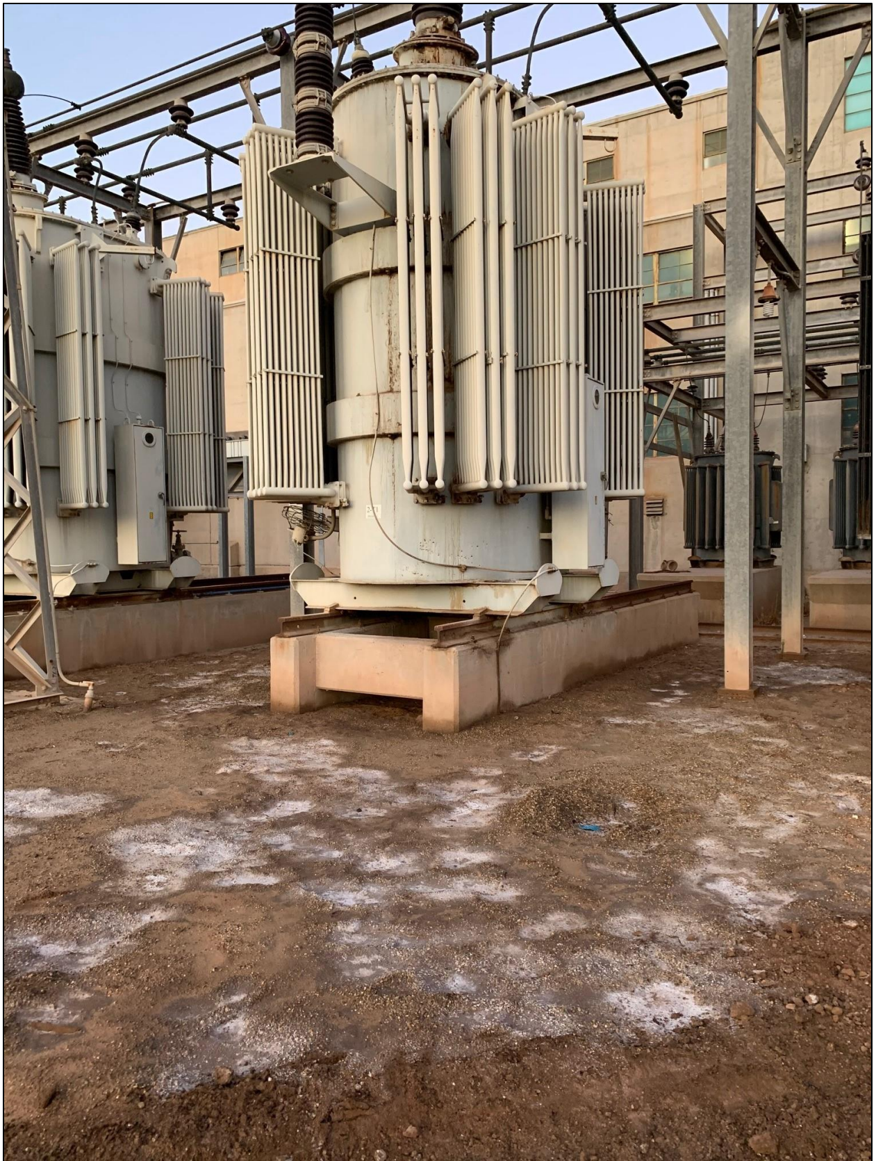
El Centro Generating Station Steam Turbine Unit 2-1 33MVA Main Generator Step-Up Transformer
