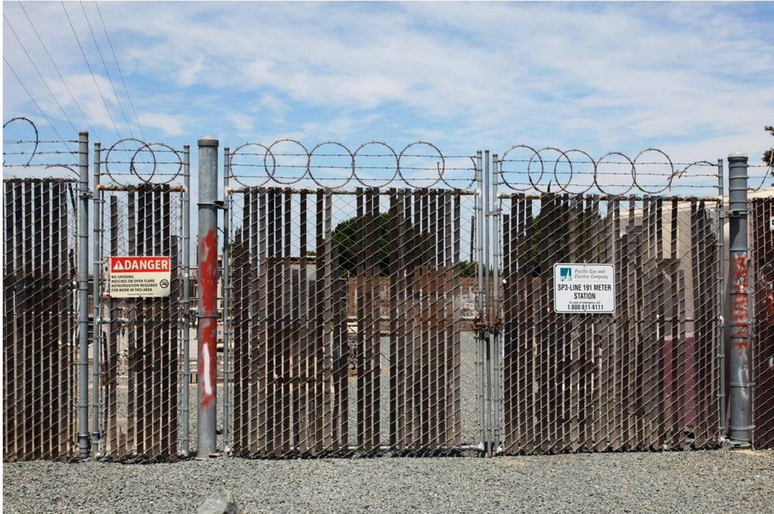
Figure 15 (continued) PG&E STANPAC3 Facility Looking North
