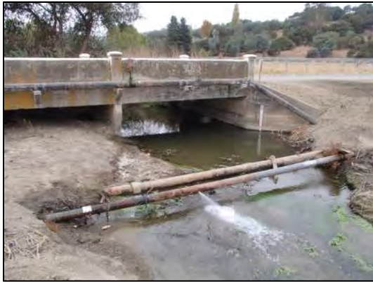
Photo 6. View looking south from the north side of Anzar Road Bridge. Note sediment accumulation under eastern span of bridge and leaking irrigation pipe on the north side of the bridge.
