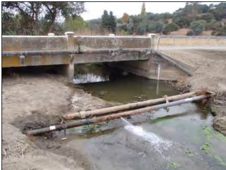
Photo 2. Pipe observed leaking water into San Juan Creek
