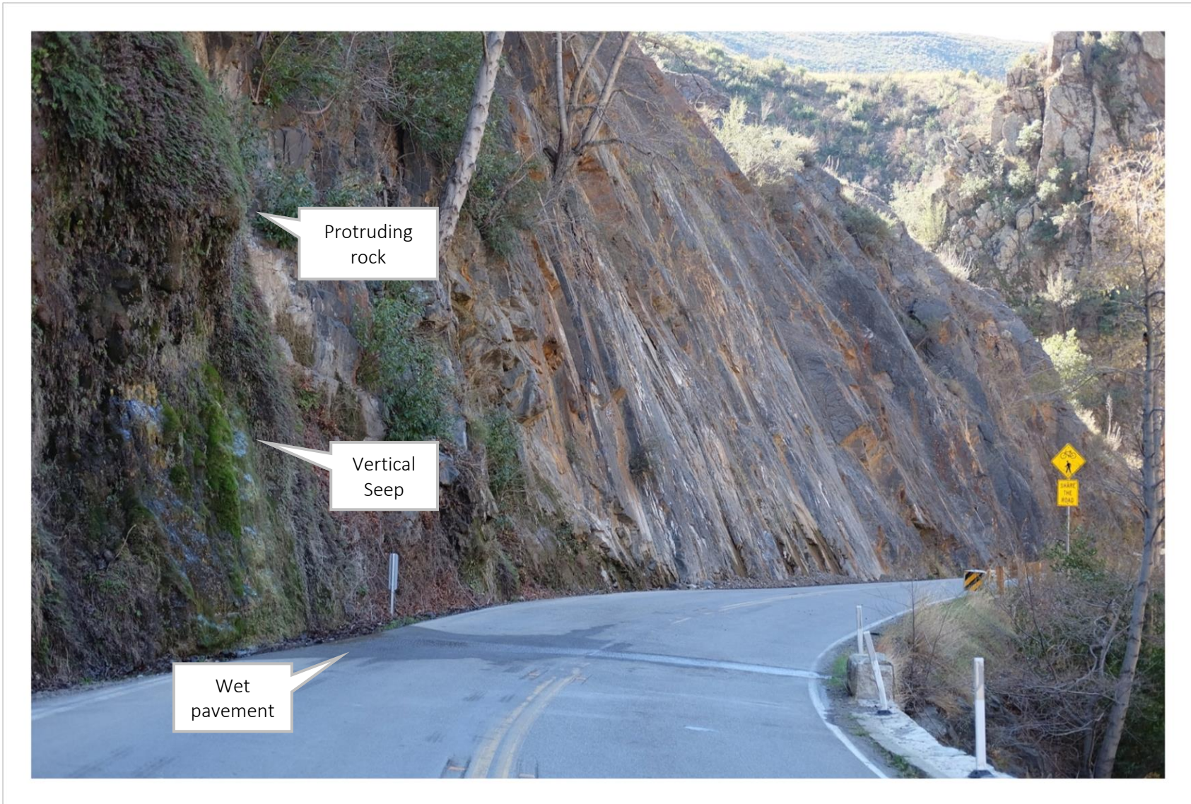
Figure 9. Wet Pavement caused by Springwater and Protruding Rock on Roadway
