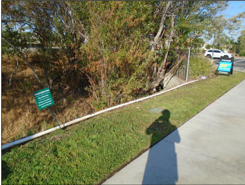
Figure 6. Earthen ditch, covered by vegetation and terminating under Margarita Road in a cement culvert. View southwest.
