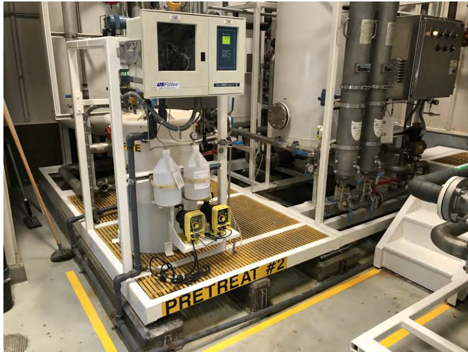
Photograph 9: Water treatment system in building B59 on Parcel 2.
