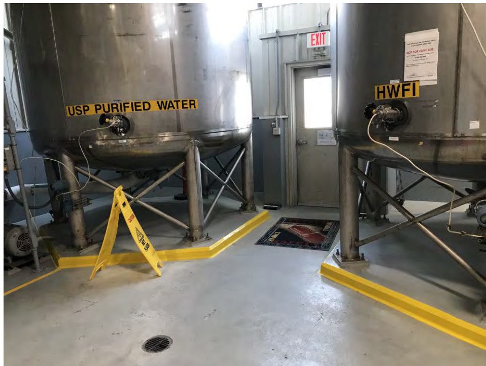
Photograph 10: Water treatment purification tanks in building B59.
