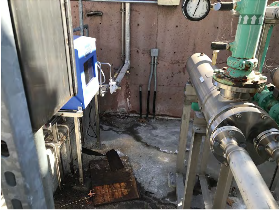
Photograph 27: Corrosion on secondary containment pump of water treatment system on exterior of building B81 on Parcel 4.
