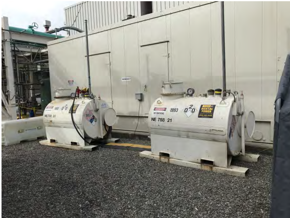
Photograph 6: Typical aboveground storage tanks on Parcel 2.
