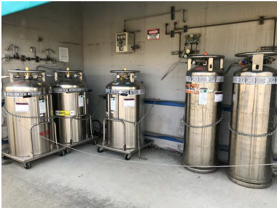
Photograph 8: Gas aboveground storage tanks on exterior of building B46 on Parcel 2.
