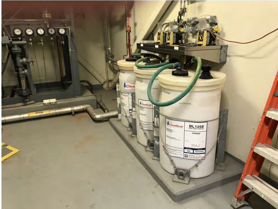
Photograph 7: Water cooling treatment system in building B44.
