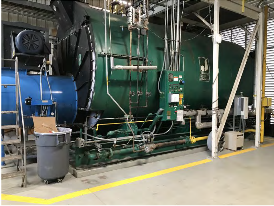
Photograph 15: Boiler in building B63.
