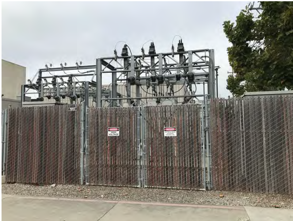
Photograph 12: Electrical substation proximate to building B61 on Parcel 2.
