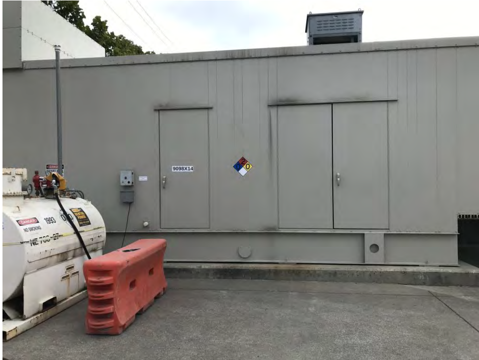
Photograph 5: Generator and aboveground storage tank proximate to building B44 on Parcel 2.
