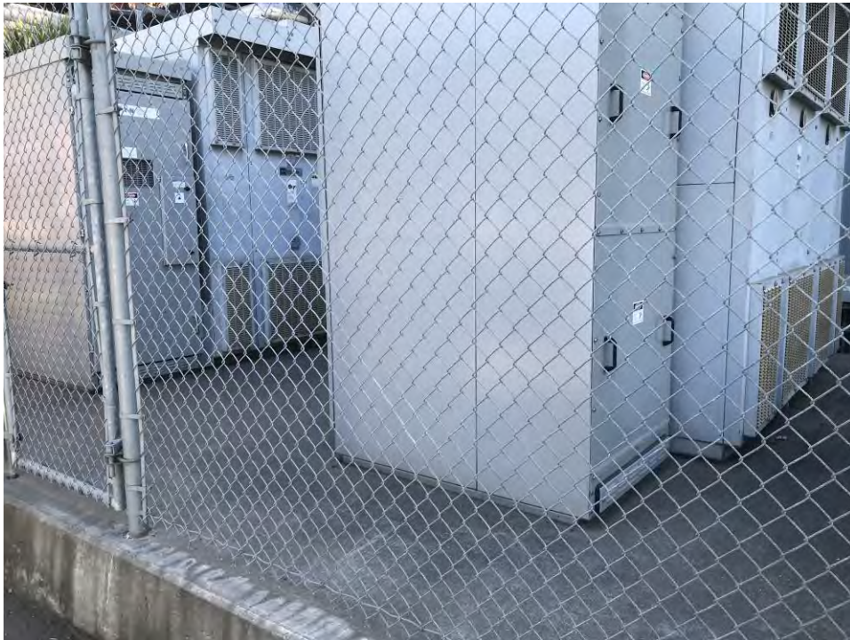
Photograph 28: Transformers proximate to building B80 on Parcel 4.
