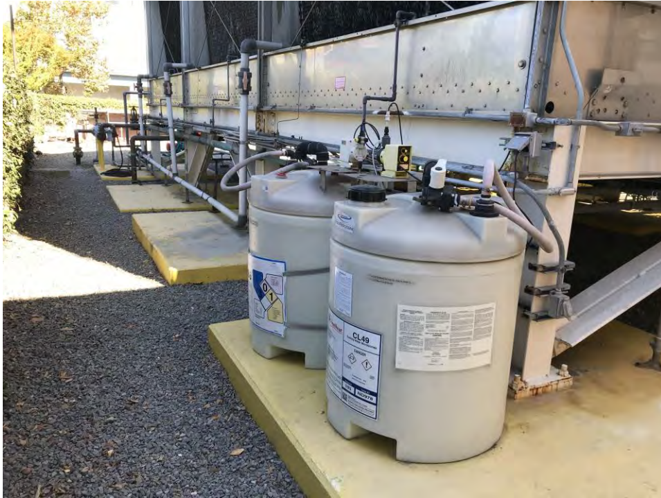
Photograph 23: Chilling system on exterior of building B82 on Parcel 4.
