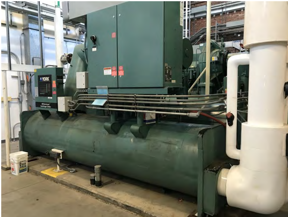
Photograph 24: Chiller in building B82.
