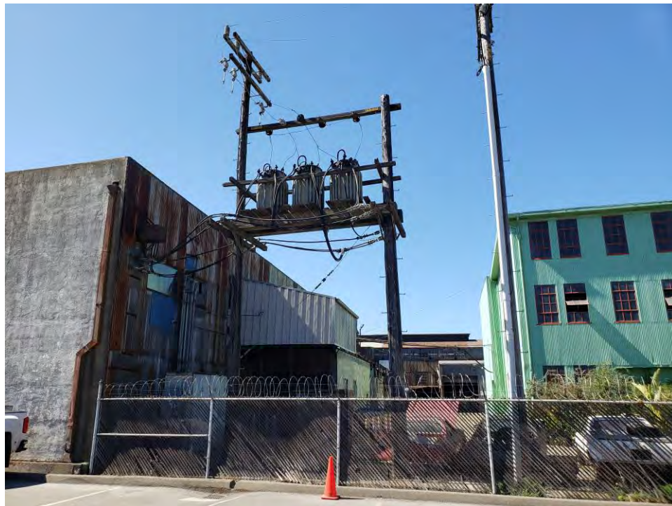
Photograph 34: Transformer on property north of Macaulay Foundry.
