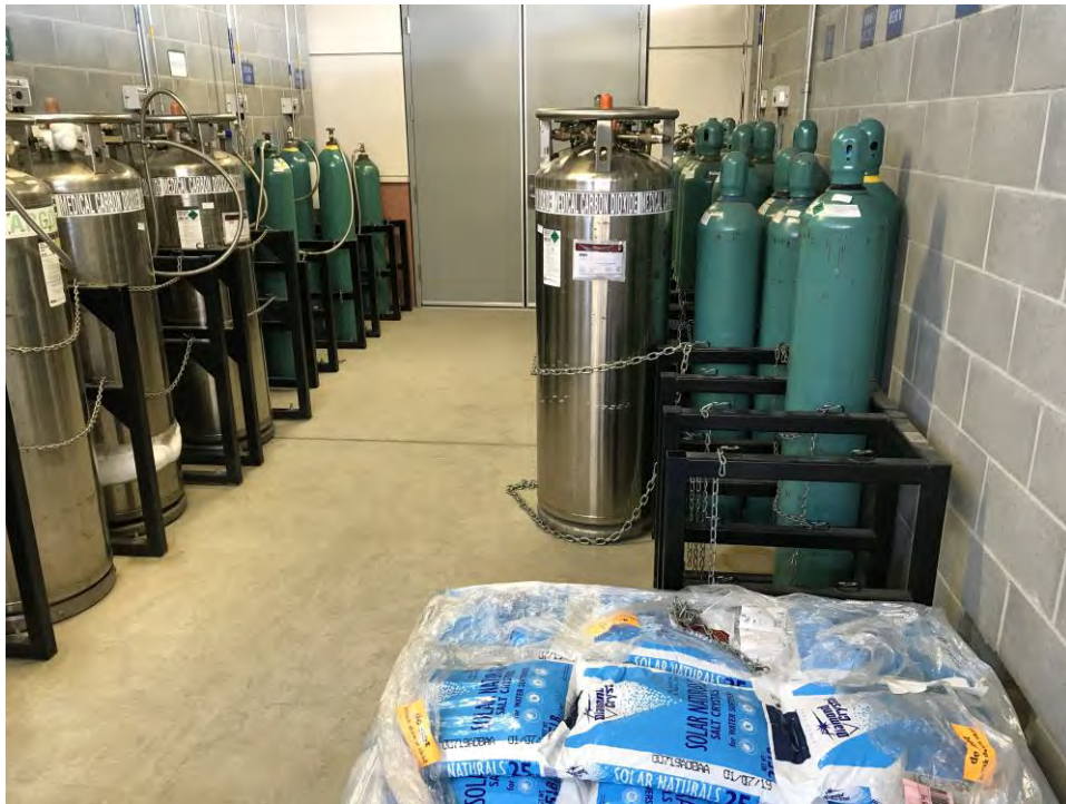
Photograph 26: Gas aboveground storage tanks in building B88.
