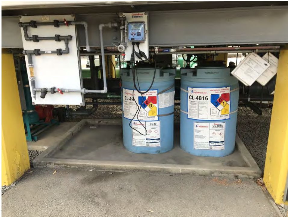
Photograph 14: Chilling equipment and chemicals on secondary containment on exterior of building B63.
