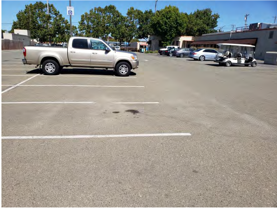
Photograph 19: De minimis petroleum staining in Parking Lot D on Parcel 2.
