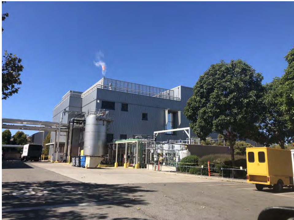
Photograph 4: Cooling tower on northern portion of Site.
