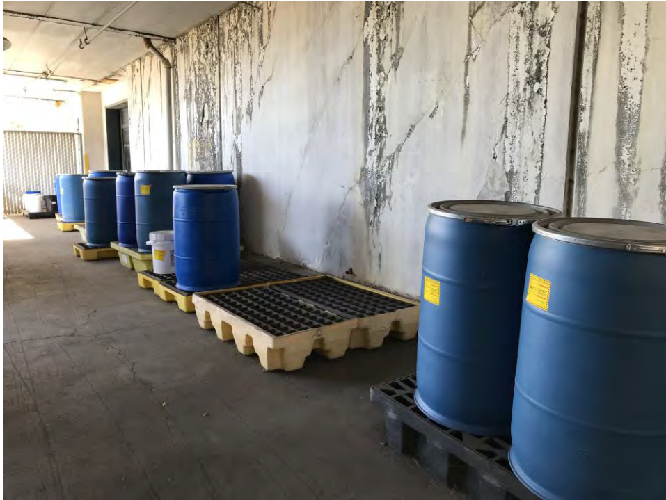
Photograph 21: Hazardous waste storage area and deteriorating paint in building B84.
