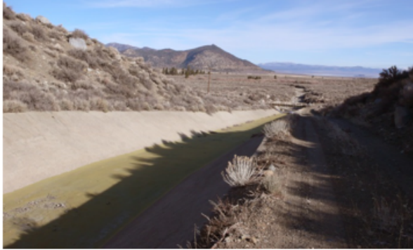
Existing concrete spillway and access road, looking south, unlined spillway in background
