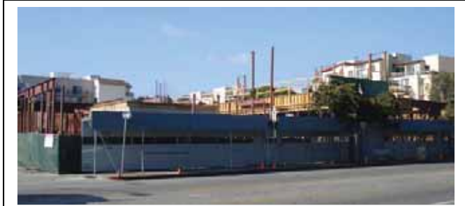
Construction activities anticipated to occur in the City would require the use of heavy equipment, generators, power tools, and other equipment, which may generate noise in close proximity to sensitive receptors, such as residences.
