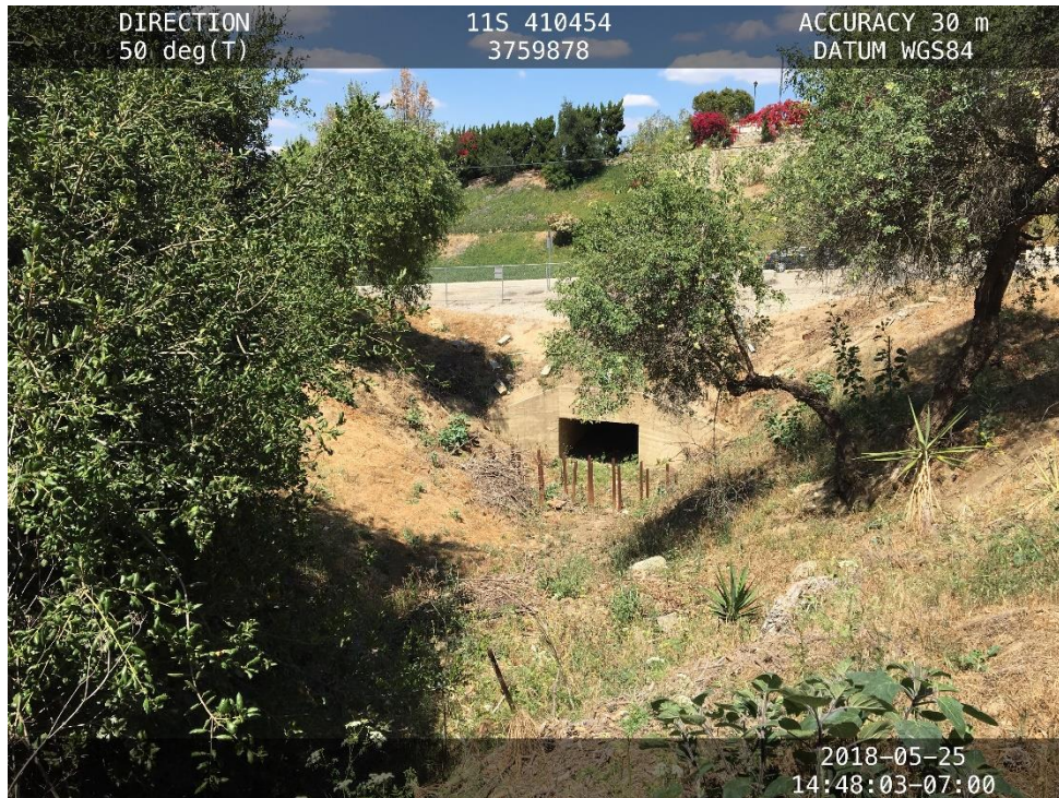
Photo 2. Depicts where Drainage 1 exits the Study Area via a culvert under South Hacienda Boulevard.
