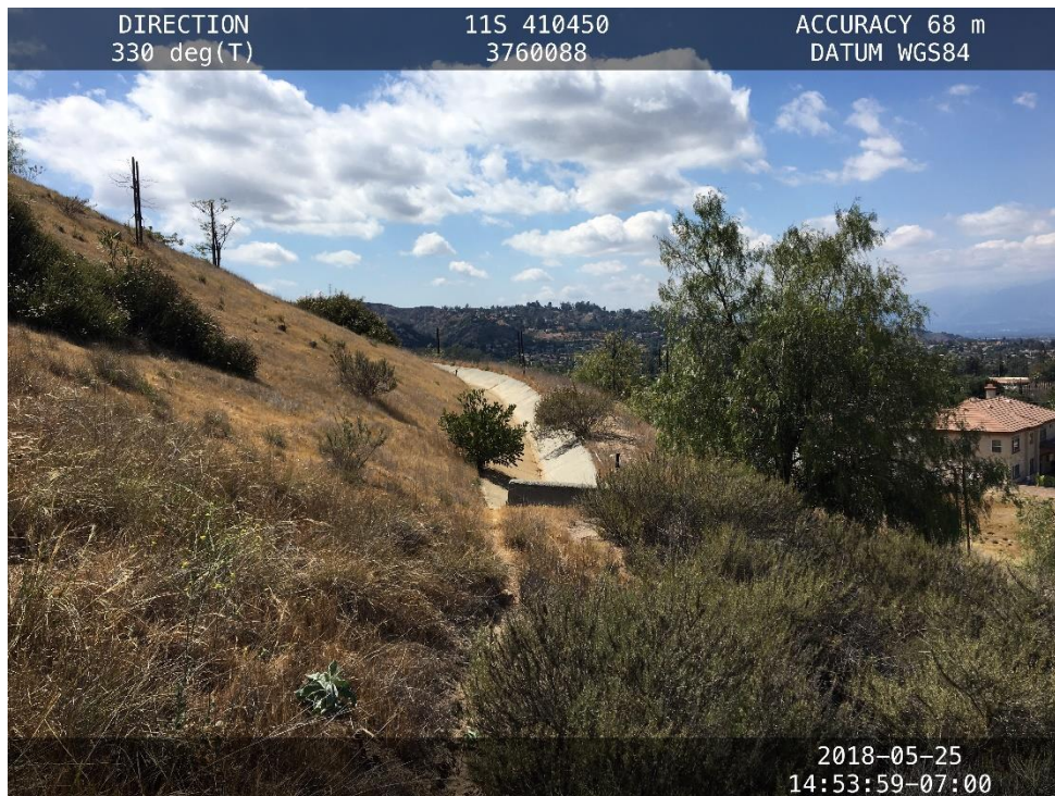
Photo 4. Depicts a concrete v-ditch at the end of Drainage 2 that directs water into a culvert at the north edge of the Study Area.
