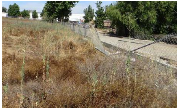
Photograph 7: Broken fence on north end of the Property.
