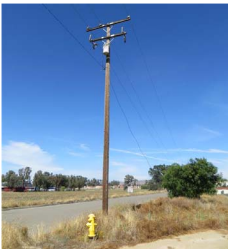
Photograph 10: Pole transformer by southwest corner of Property or possibly fronting west adjoining site.
