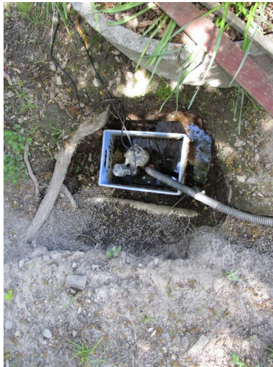
14. Sump pump adjacent to the office
