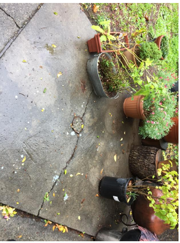
Photo 8: View of abandoned well casing at 376 Yolanda Avenue
