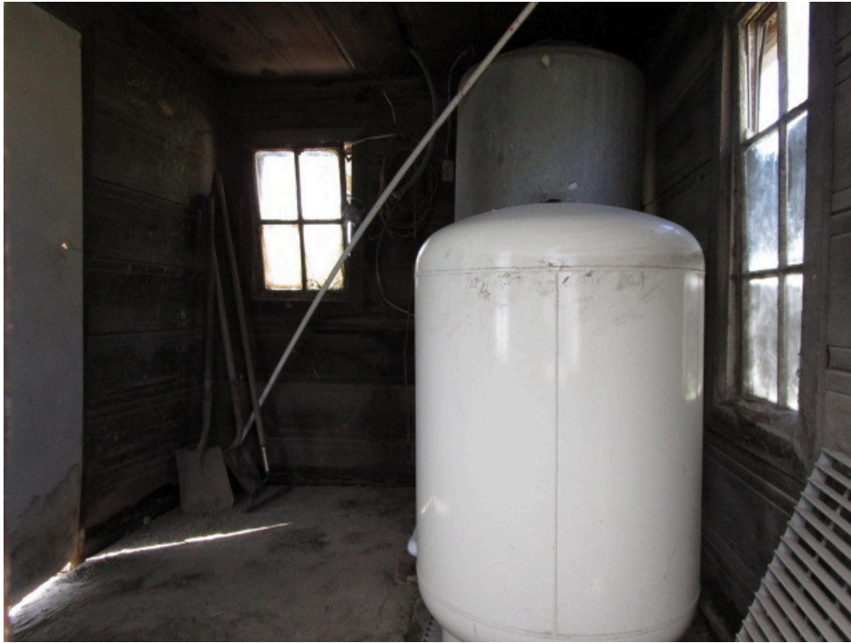
41. Apparent pressure tank in the shed
