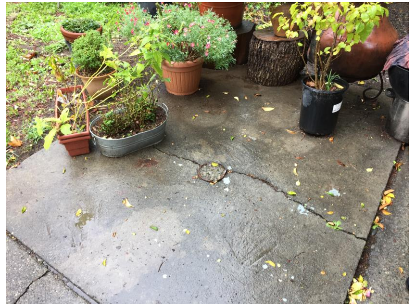
Photo 8: View of abandoned well casing at 376 Yolanda Avenue
