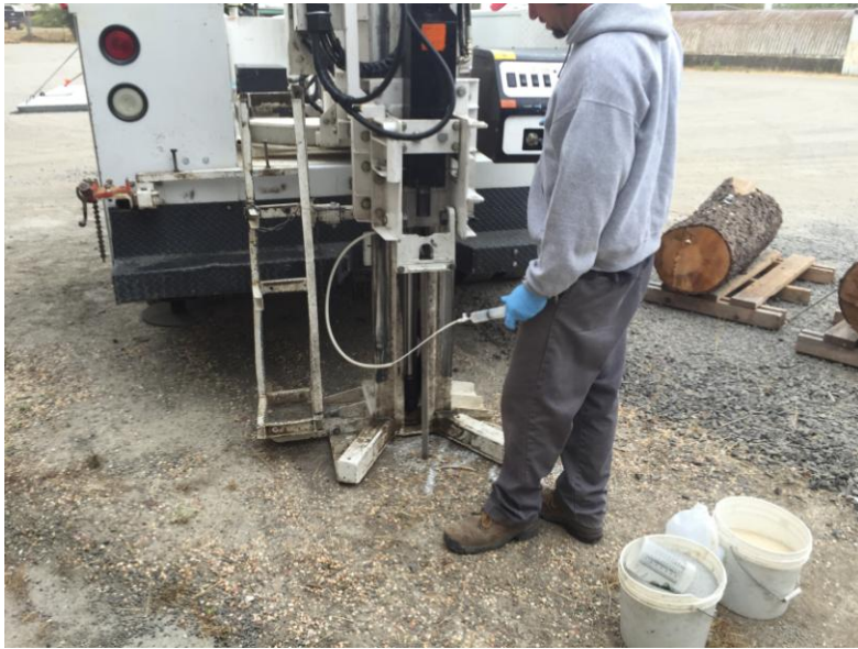
Photo 1: View of TEG advancing soil probe with 1-inch direct push rod, testing soil pressure, granular BenSeal and sand on right
