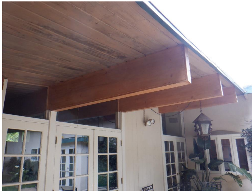
Detail of exposed roof rafters in the wide eave overhangs, clerestory windows, and hanging Spanish style lantern.
