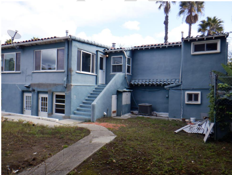
Exhibit 30. West façade with variations of windows and three entries. This photograph shows the two major additions to the house. The original southwest corner of the house is at the top of the staircase with an addition to the west and another on the south.
