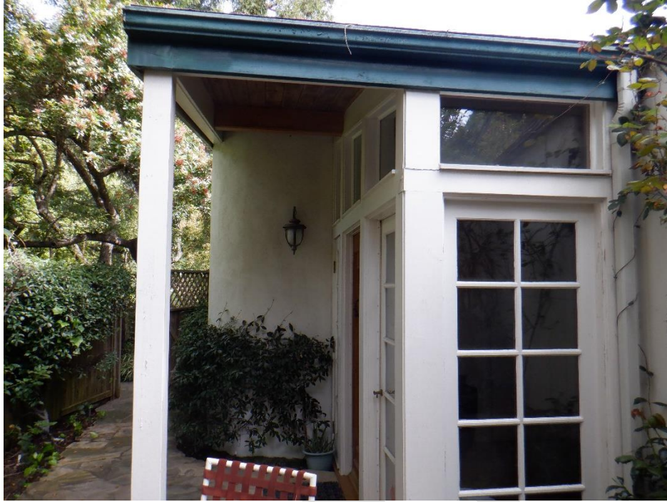
Exhibit 15. Front entry courtyard with recessed door on west façade, looking north. According to building permit records, the front entry was expanded and the windows were added in 1998.
