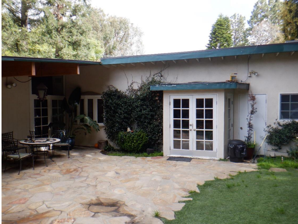
Detail of exposed roof rafters in the wide eave overhangs, clerestory windows, and hanging Spanish style lantern.
