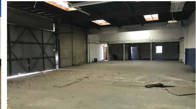
Photograph 6. View inside the former automotive repair building present on the southern portion of the subject property.
