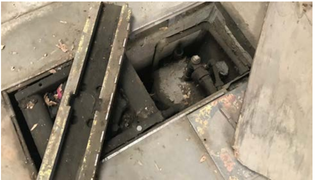
Photograph 7. View of the in-ground hoists present inside the former automotive repair building on the southern portion of the subject property.
