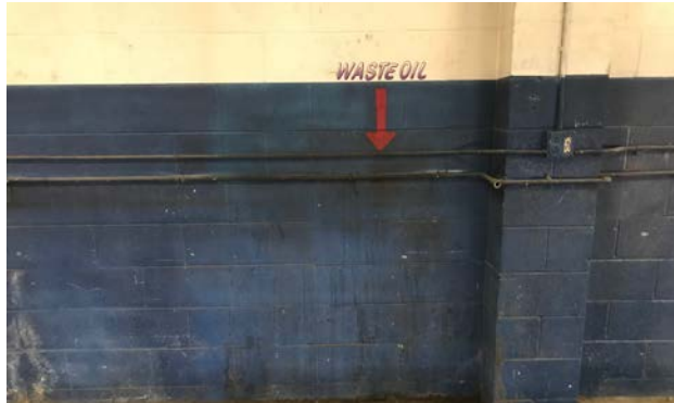
Photograph 8. View of the "waste oil sign" inside the former automotive repair building on the southern portion of the subject property.
