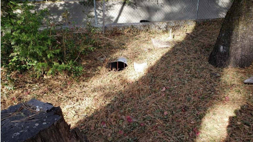
Photo 11. Photo depicts a 24-inch corrugated metal storm drain inlet from area north of site into concrete-lined channel.
