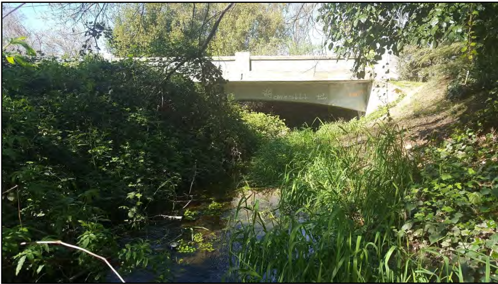
P02: Standing in Clover Creek looking north at the First Street Bridge to be replaced.
