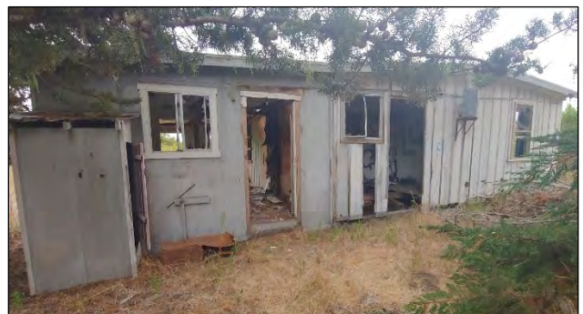
Photo 6: West elevation of the residence with addition on the left, view facing east.
