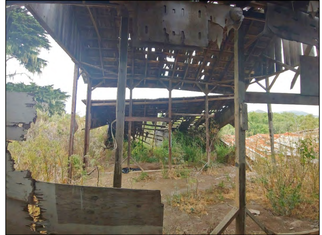
Photo 11: View from south crib barn interior, across barn, to north crib. View facing north.
