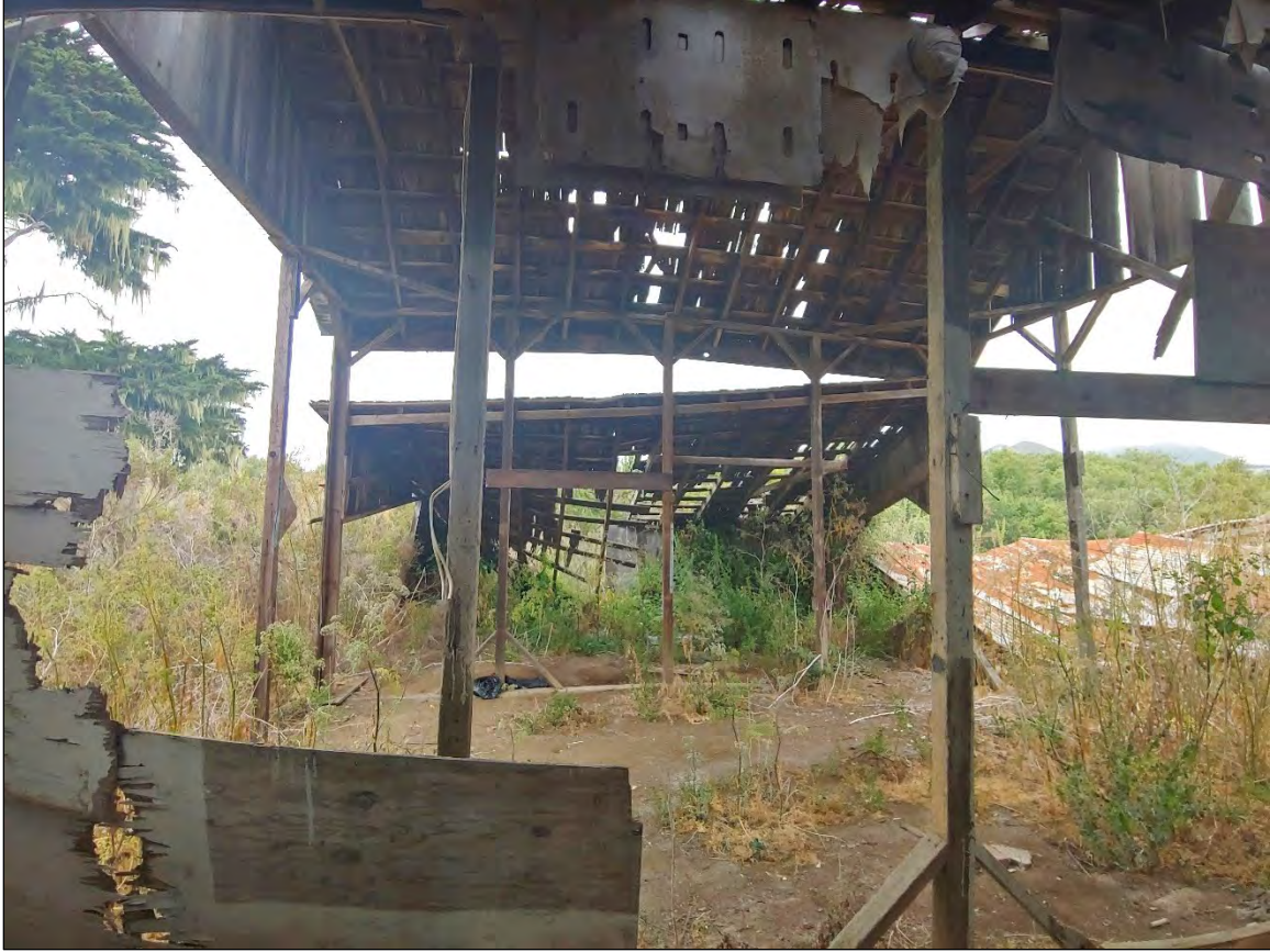
Figure 5-8 View from south crib barn interior, across barn, to north crib. View facing north.
