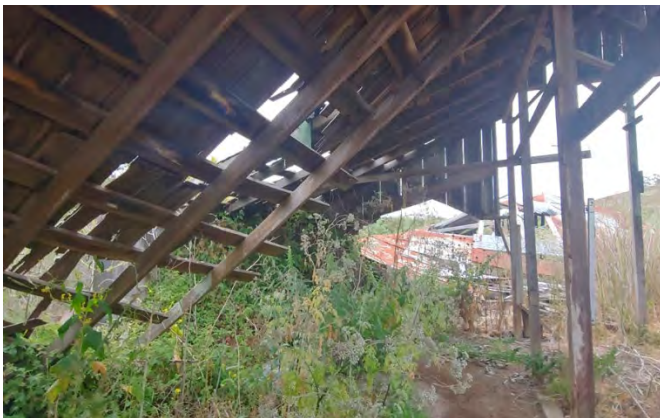
Photo 10: Crib on north side of barn interior, view facing east. Unknown collapsed building in the background.
