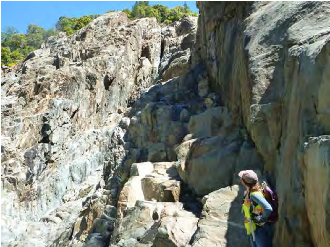
Close up of shear zone in existing spillway discharge channel. See above photograph for location of person (red oval).
