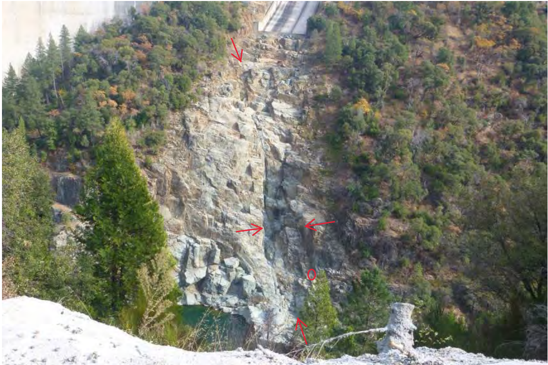
Existing spillway and discharge channel. Note jointed rock mass and deep erosional slot coincident with ancient shear zone (between arrows). Approximate Secondary Spillway alignment shown by black line. Red oval marks approximate location of person in photograph below.
