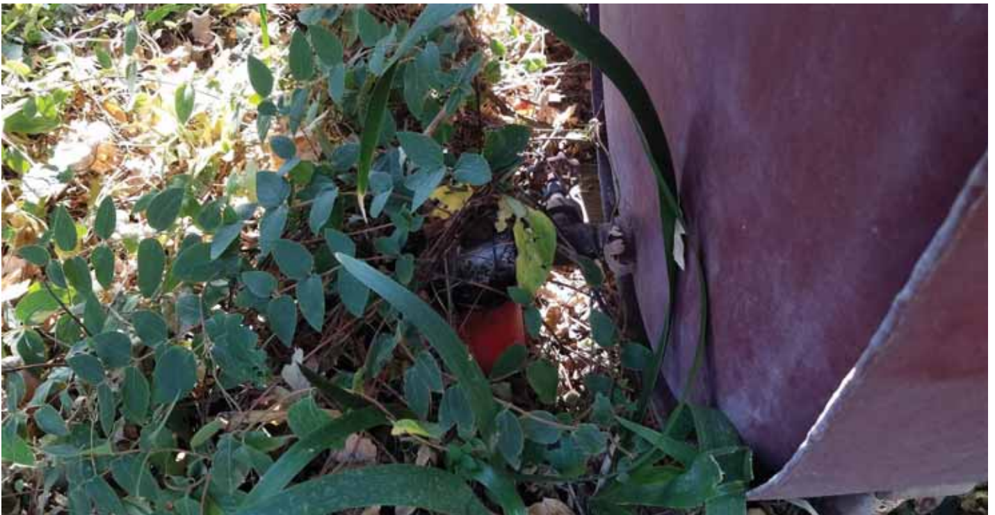
Photo 4: East side of heating oil tank where fuel is piped toward the residence.
