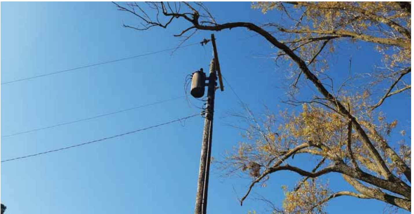
Photo 18: Pole-mounted transformer located southwest of former western residence.
