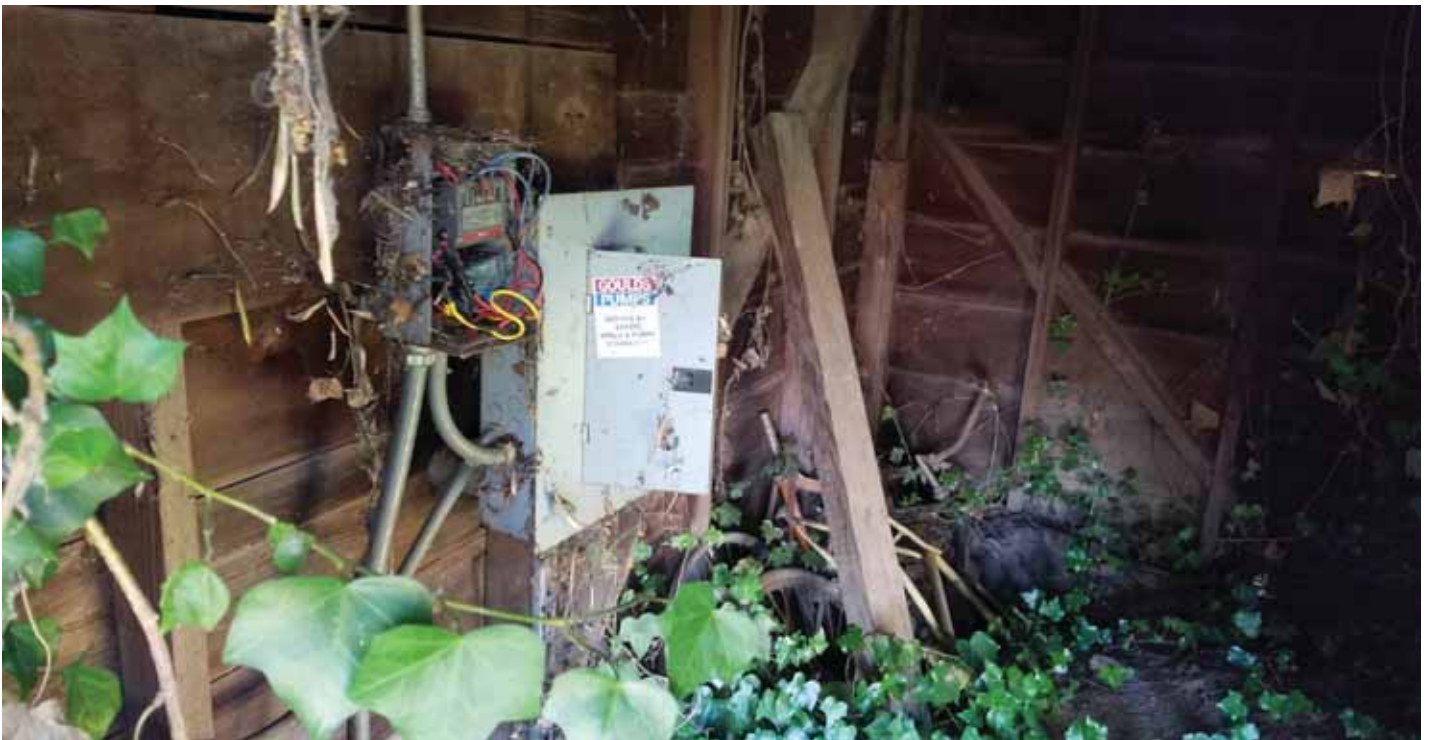
Photo 16: Interior of the well house with electrical breaker box.
