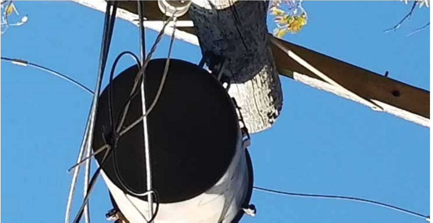
Photo 19: Pole-mounted transformer depicted in previous photos. No signs of leakage.
