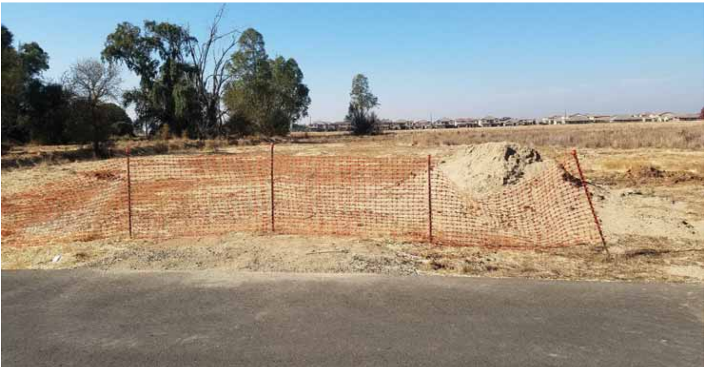
Photo 24: Area along Lousada Drive where utility sand has been temporarily stored during construction on the eastern adjoining residential development.
