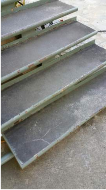
Main stairs have open risers.
