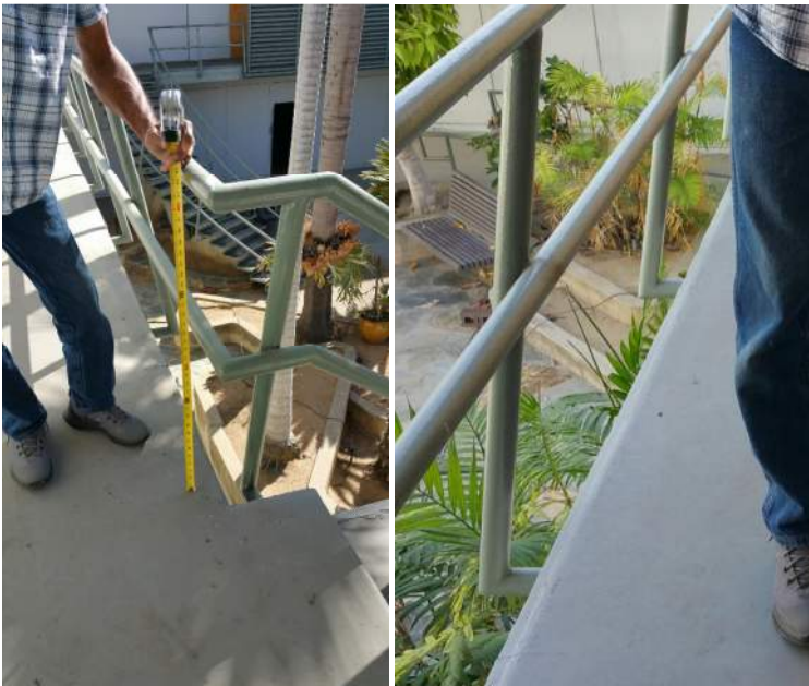
The balcony guard rail height and the lack of the edge protection.
