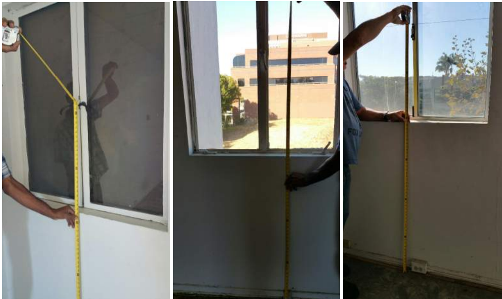
Second floor steel window’s latch is mounted at 62” above the floor.
