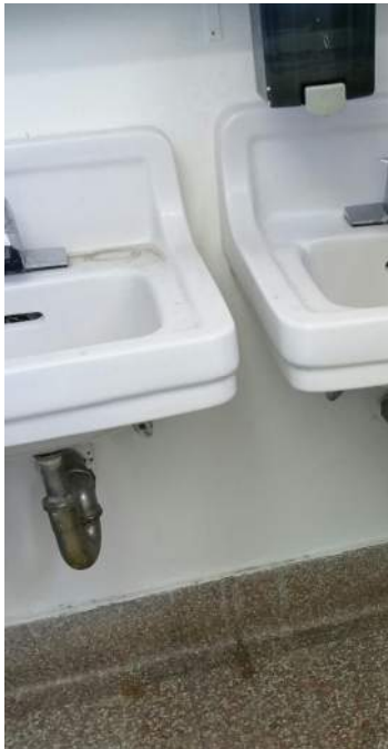
There is no insulation for the water supply and the drain pipes.
