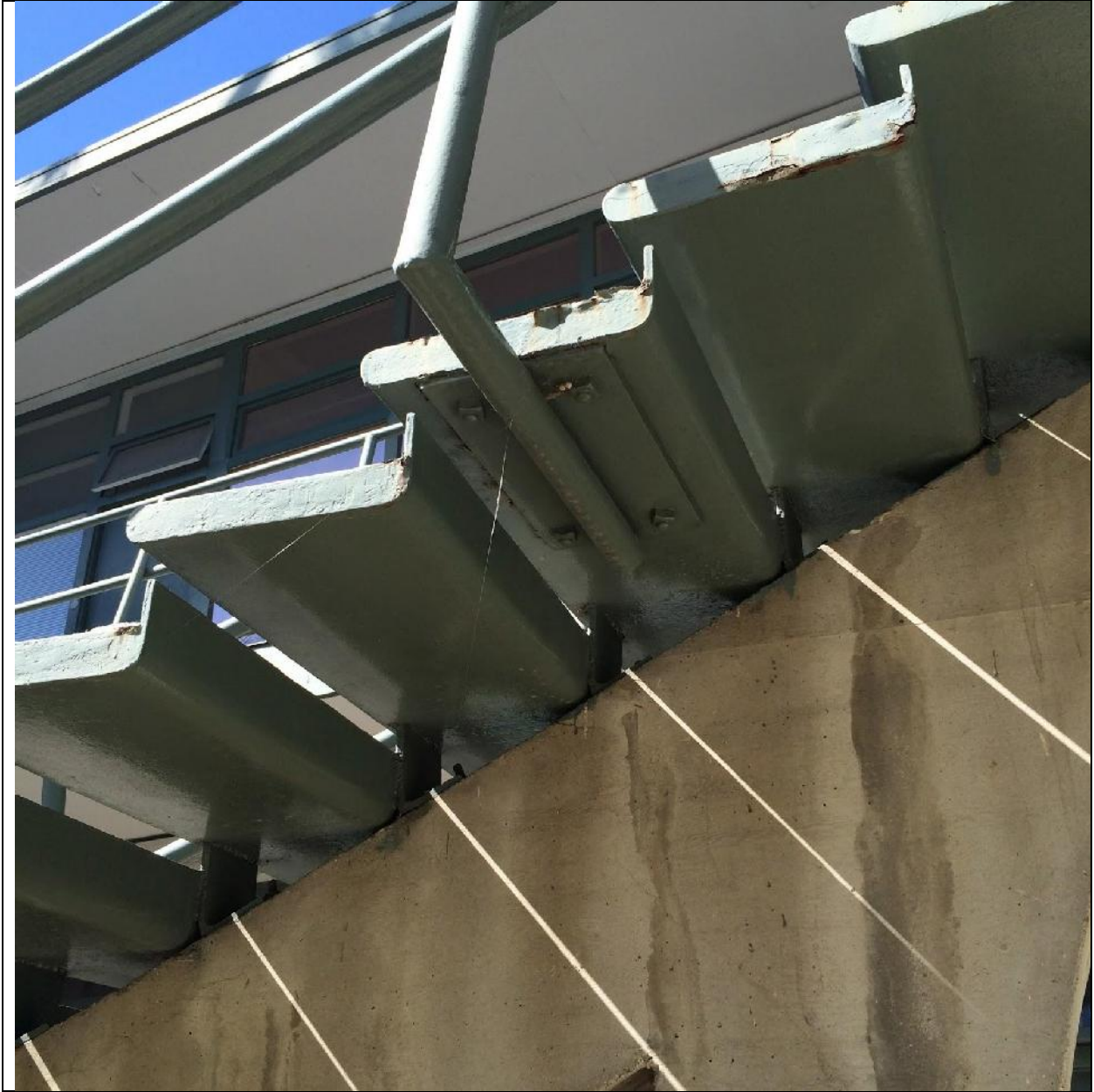
Stairs (Photographic Study) Continued - Above: The stairs are cantilevered from a central concrete spine.
