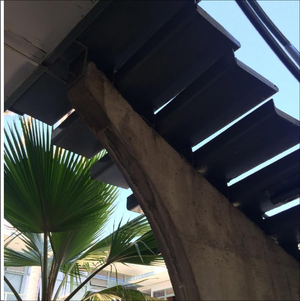
Above: The stairs are cantilevered from a central concrete spine. (photo by Laura Clayton Baker)
