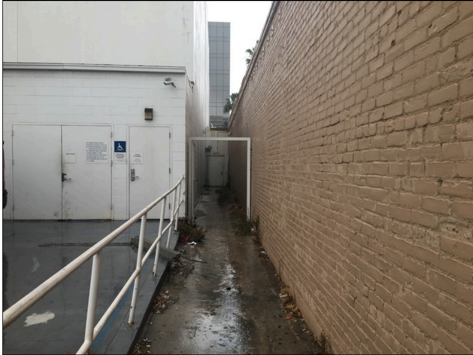
Photo 21: View of northern concrete-paved walkway on the southwest portion of the subject property looking northeast.
