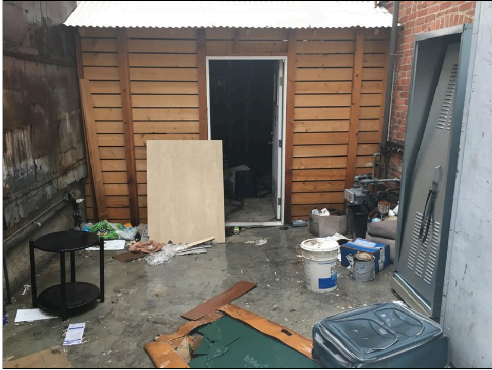
Photo 17: View of canopy and storage area on the central portion looking northwest.
