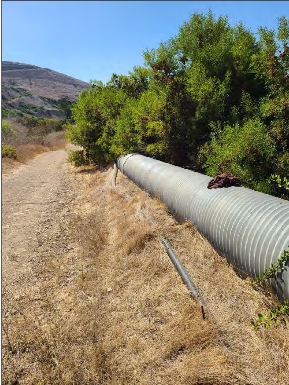
Photograph 7. View of abandoned storm water retention system.
