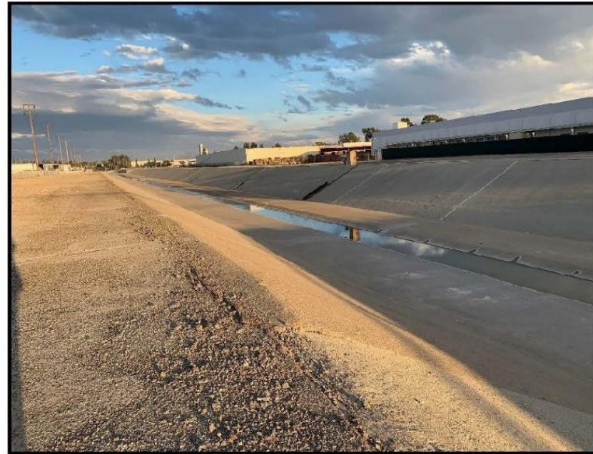
Photo 1: Representative photo of the concrete-lined channel land cover (Coyote Creek Channel) and dirt maintenance road. This section is located in Segment O.
