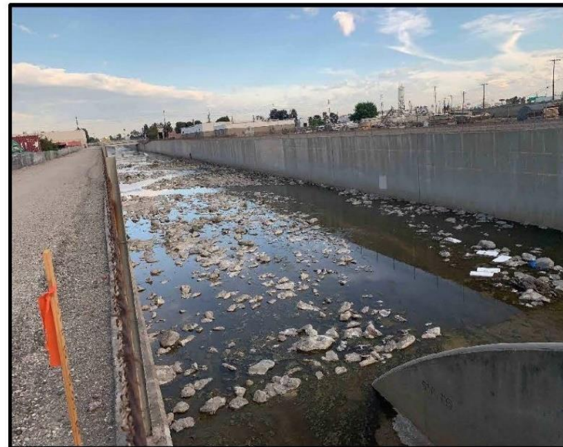
Photo 2: Representative photo of the concrete-lined channel land cover (Coyote Creek Channel), this section is located in Segment P.
