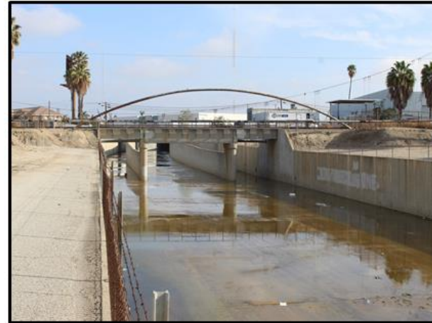
PHOTO 10: View looking northeast of the Union Pacific (UP) railroad and gas utility pipeline.
