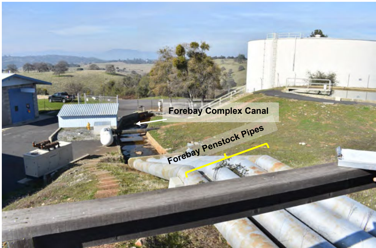
Figure 18: Forebay Penstock Pipes and Canal
