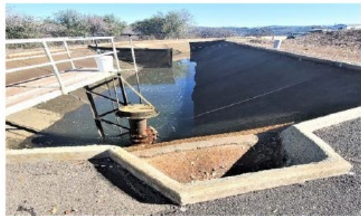
Photo 6 - Sedimentation basin - drained for cleaning
