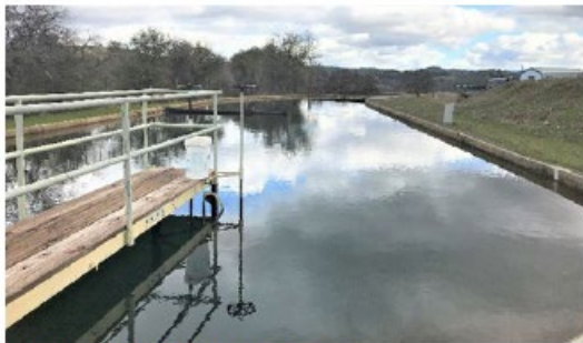
Photo 5 - Sedimentation basin outlet
