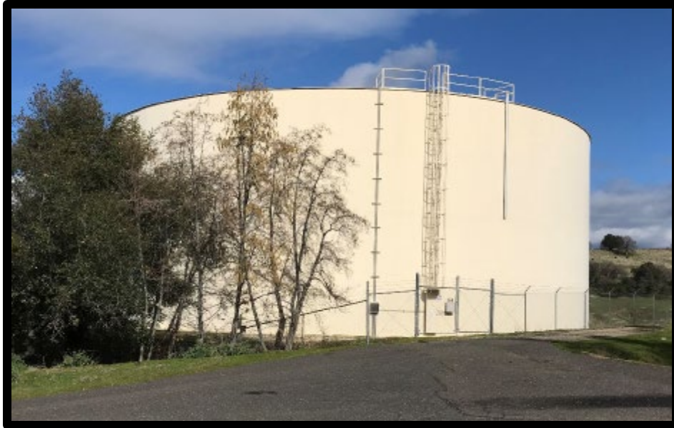
Figure 6: 2.5 MG Storage Tank
