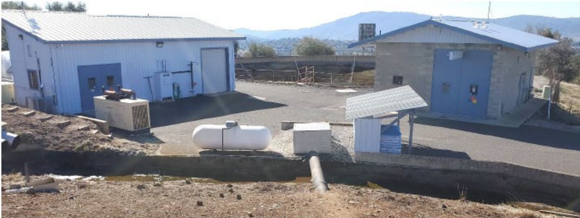
Photo 7 - Filter Building (L), clear well (background), chlorine building (R), inlet pipe to filters (foreground)
