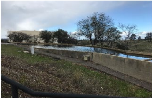
Photo 4 - Flocculation to sedimentation basin transition
