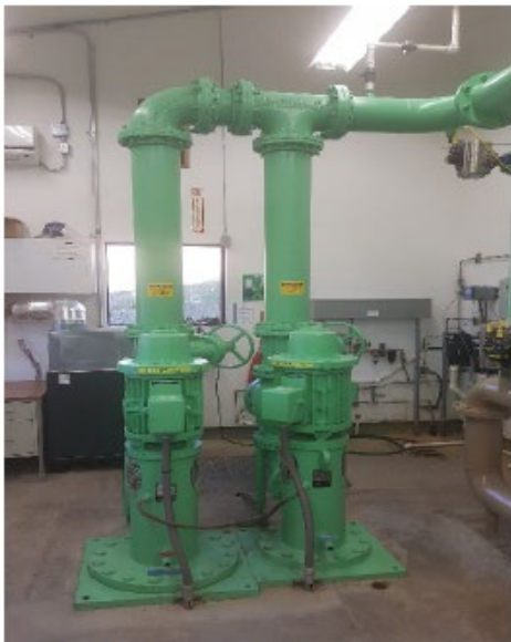
Photo 8 - Two of four filter pumps
