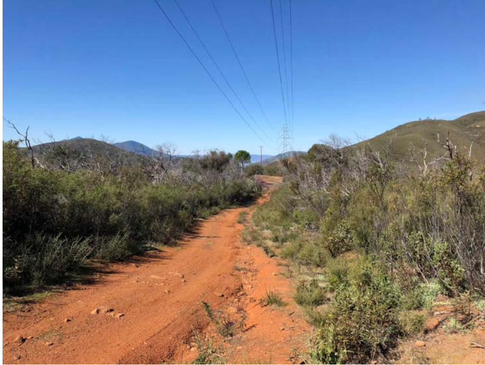
Existing PG&E access road and proposed route for power and fiber-optic cable (undisturbed habitat on right side of photo). View looking west.
