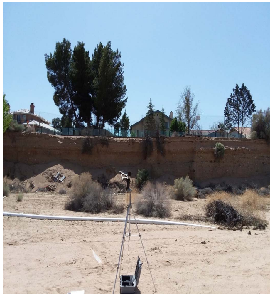
JN 6602a STNM2 looking South East. Yates Road passes along top of embankment.
