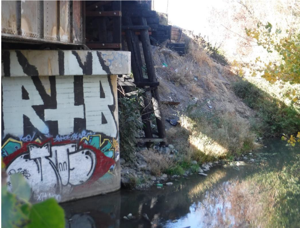
Photo 4: Failing channel protection on northeast embankment.
