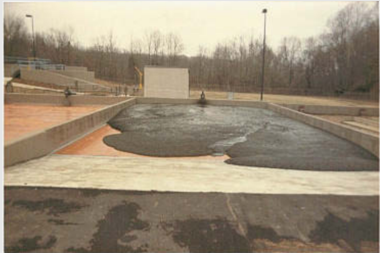
Hohenwald, Tennessee Wastewater Treatment Plant - Two 1000 square foot Wedgewater™ Filter Beds
