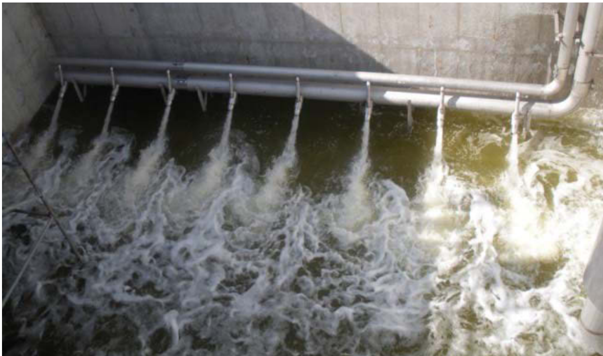
Stainless steel jet aeration header
