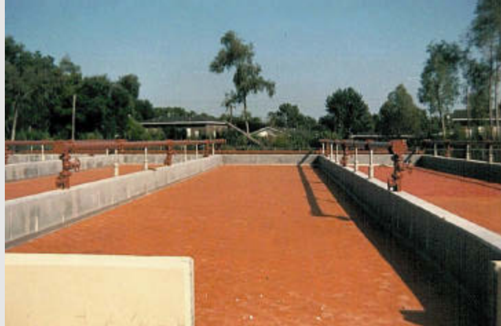
La Place, Louisiana Wastewater Treatment Plant — Four 1800 square foot Wedgewater™ Filter Beds
