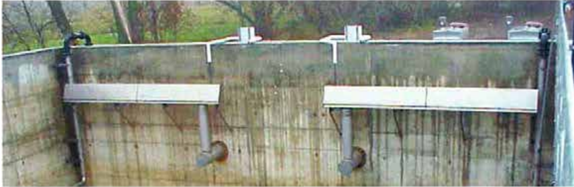
Dual stainless steel fixed air-sealed decanters
