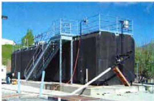
ISAM™ Packaged Sequencing Batch Reactor
