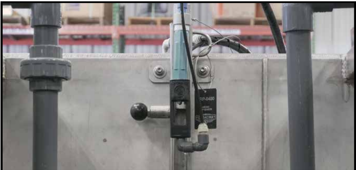
Example Sensor Installation
