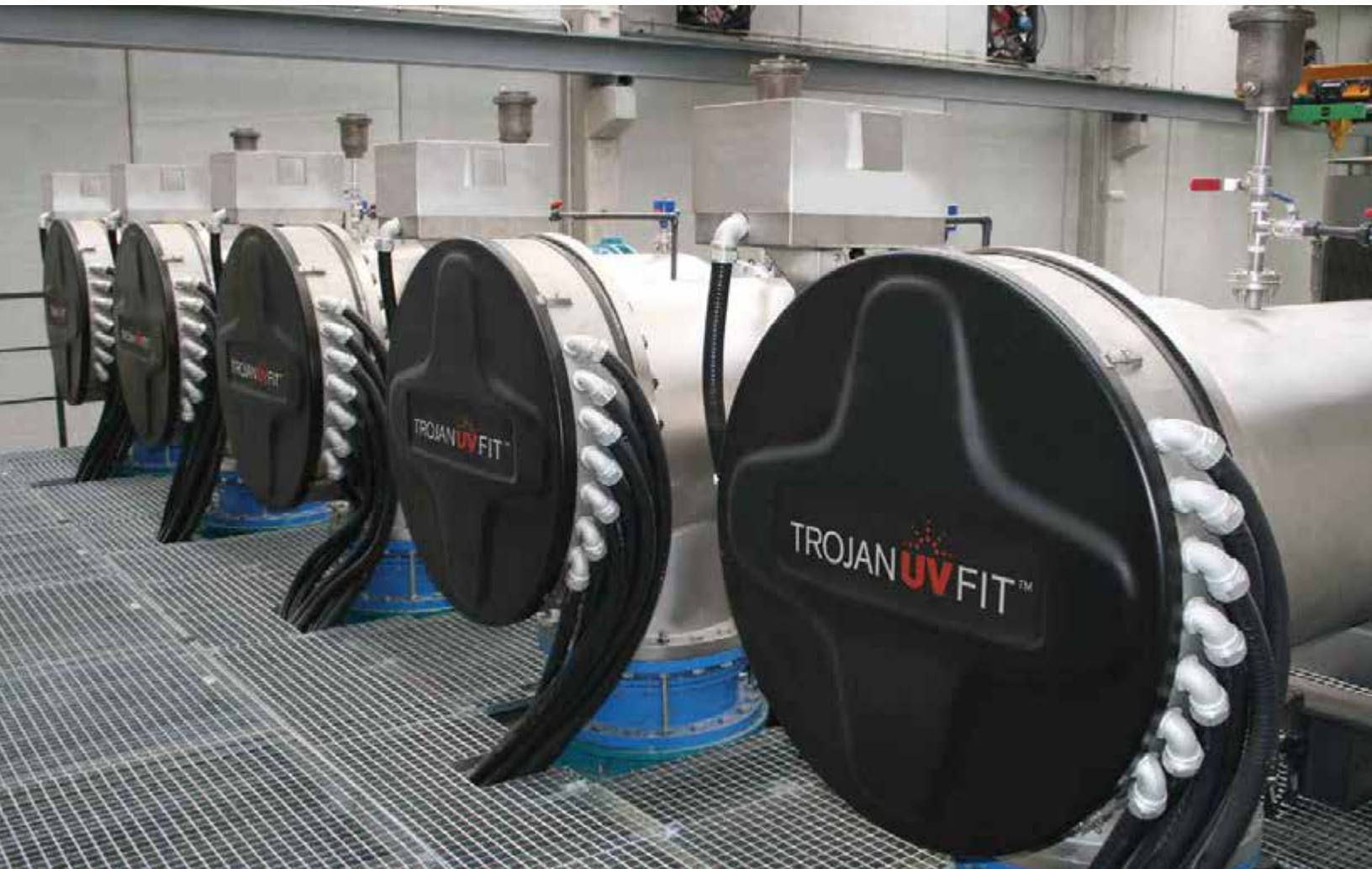
WASTEWATER DISINFECTION FILTERED IN-PIPE TREATMENT
