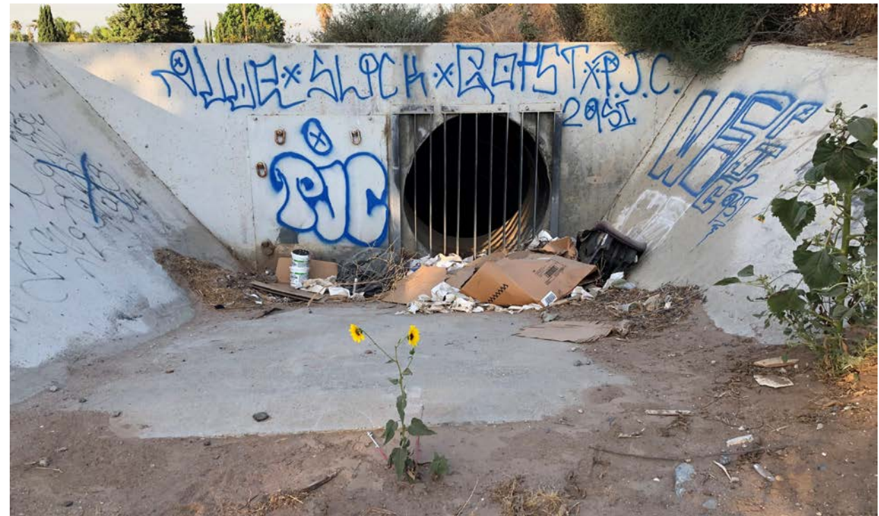
Photograph 8: Downstream view of West Riverside Canal at 28 th Street. Culvert discharges to storm drain and does not flow through to downstream segment of canal.
