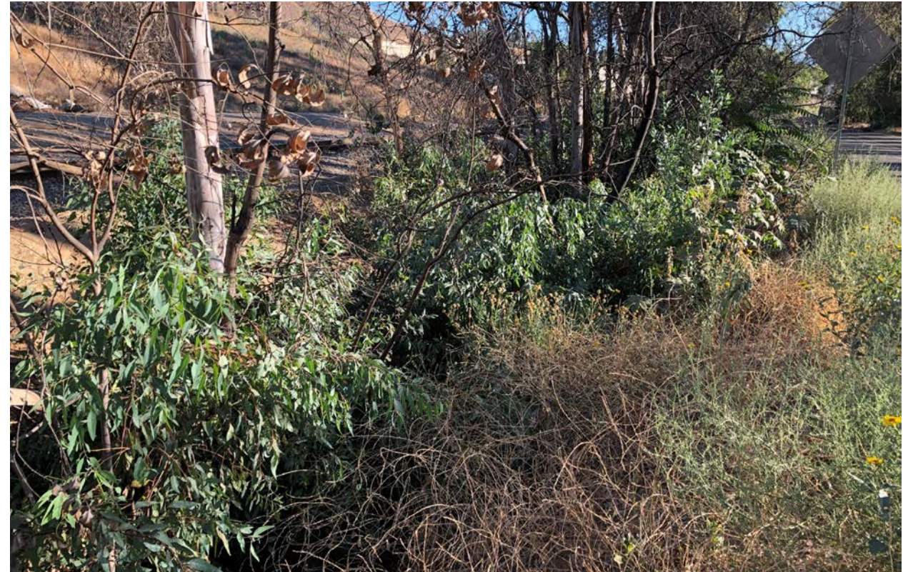
Photograph 10: : Offsite upstream view of West Riverside Canal east of 20 th Street. Note dense eucalyptus trees within abandoned canal.
