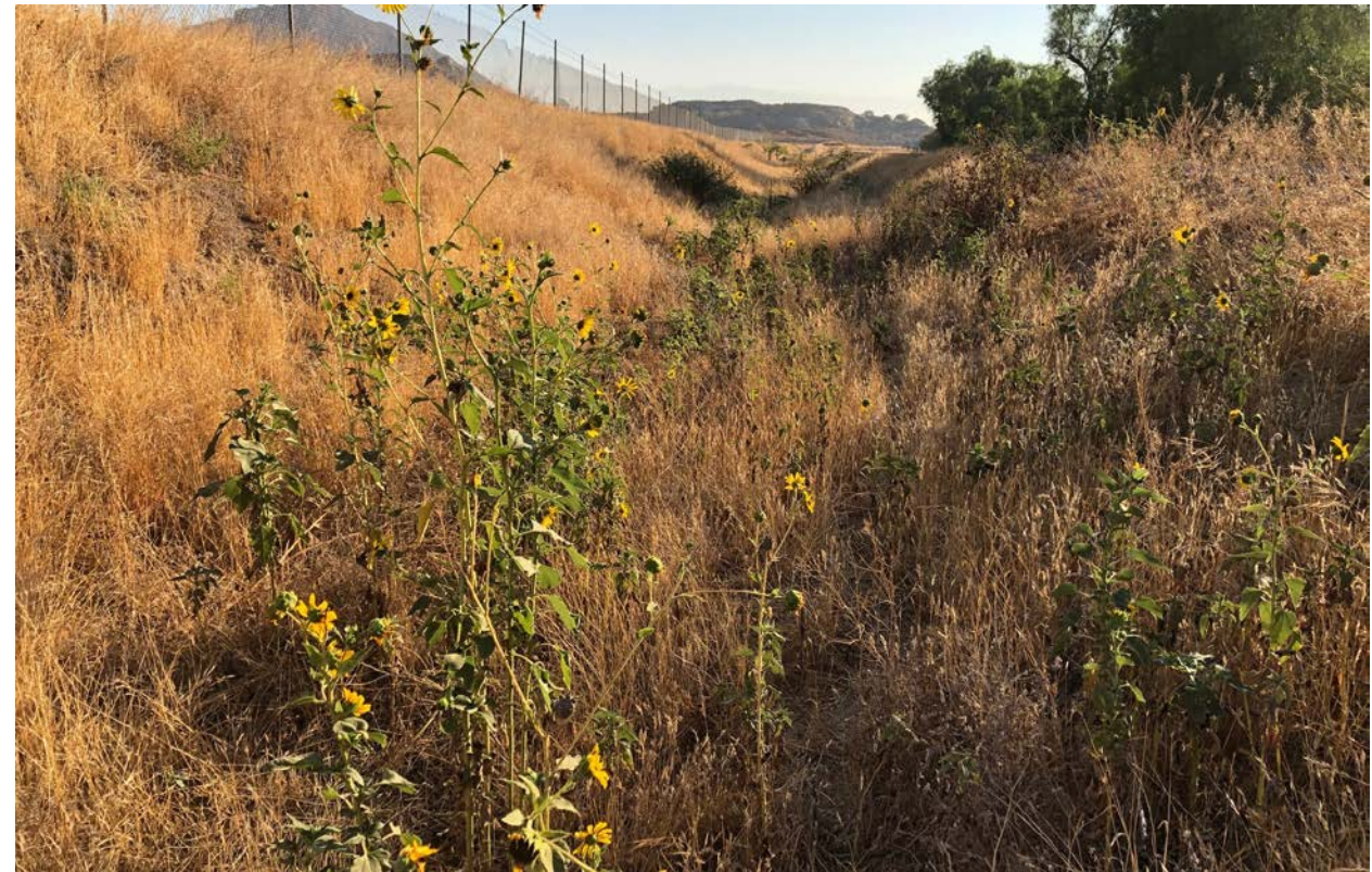
Photograph 6: Upstream view of West Riverside Canal Between 28 th and 26 th Streets. Note dense upland vegetation within abandoned canal.
