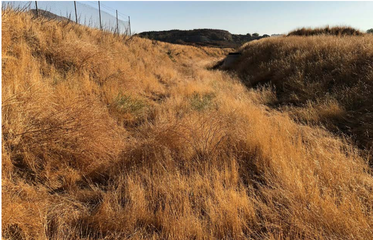
Photograph 5: Upstream view of West Riverside Canal Between 28 th and 26 th Streets. Note dense upland vegetation within abandoned canal.
