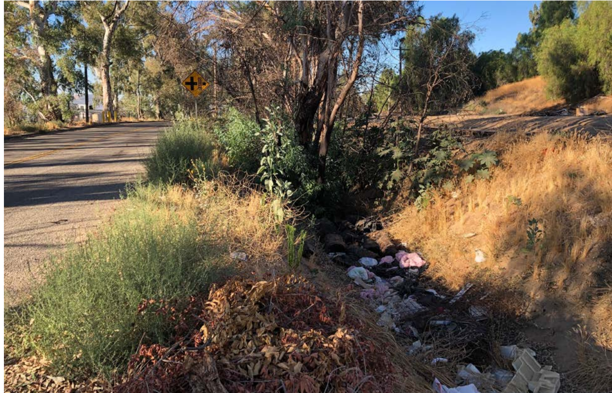
Photograph 9: Offsite downstream view of West Riverside Canal east of 20 th Street. Note trash, debris and upland vegetation within abandoned canal.
