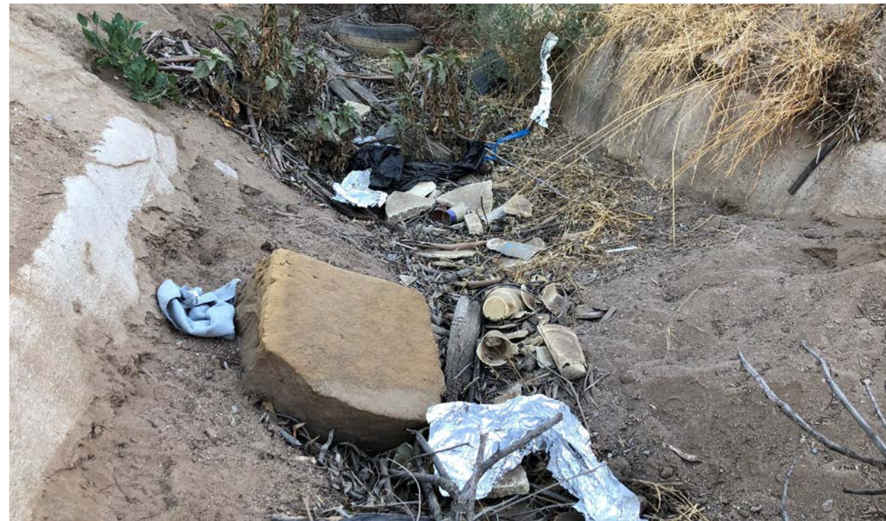
Photograph 11: Offsite upstream view of West Riverside Canal west of 20 th Street. Note trash, debris within abandoned canal and concrete sides of canal.
