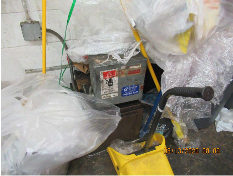
15. Loading dock plate hydraulic equipment.
