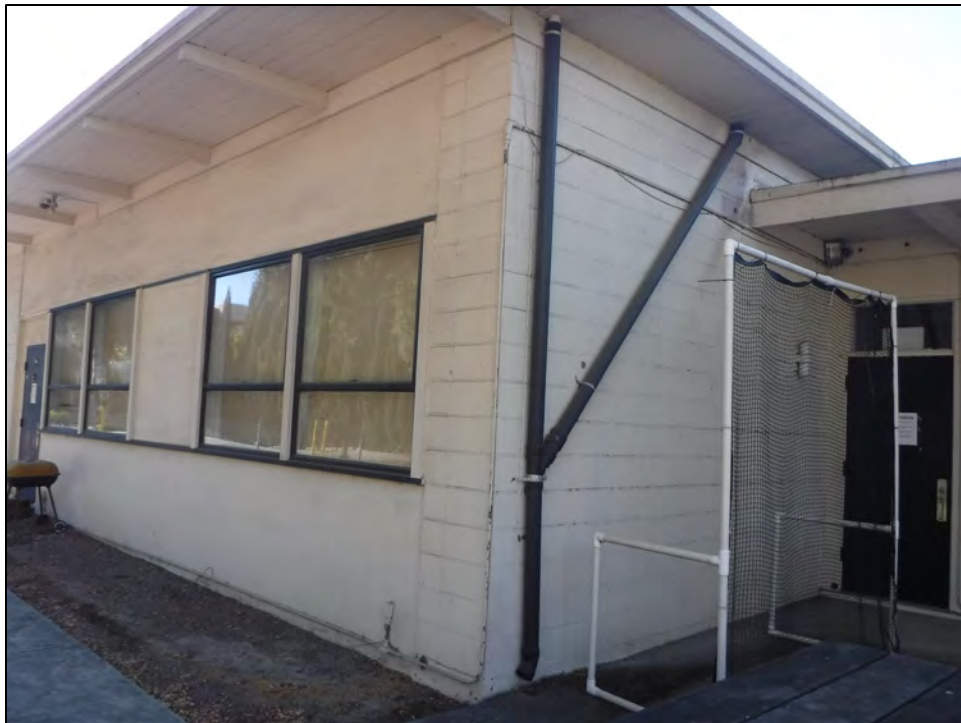
Photograph 9: Northeast corner of south building section. Note the stack-course concrete masonry units, camera facing southwest, September 23, 2020.
