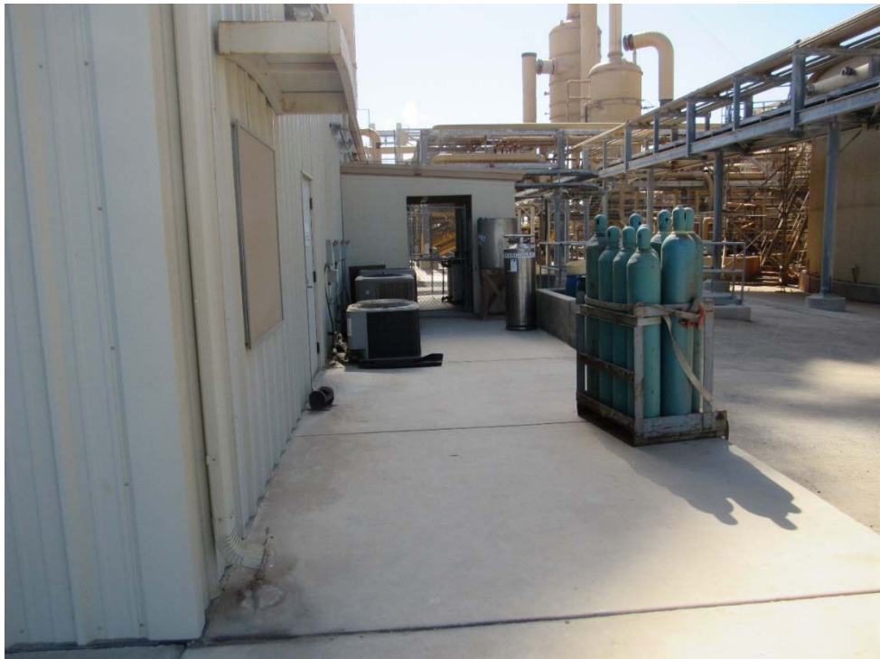
Photo 2: Looking along the south side of the control building at the HVAC units, and Argon gas cylinders.
