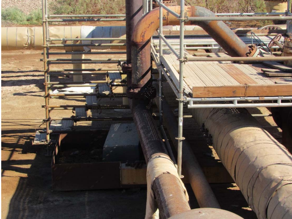
Photo 73: Looking at a secondary containment bin located under the vales at the pipe crossing road.
