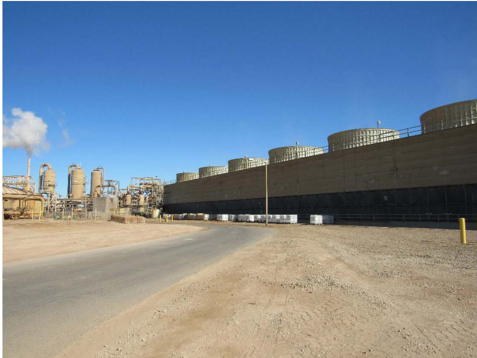
Photo 57: Looking at multiple cooling tower chemical storage containers at the west side of the cooling tower.
