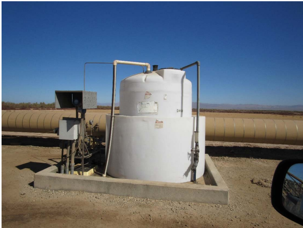
Photo 78: Looking GEO906 geothermal treatment liquid container located at the well pad.
