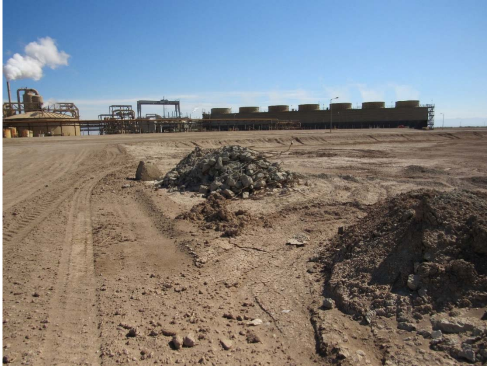
Photo 51: Looking north along the west side of the stormwater retention basin at a concrete debris pile.
