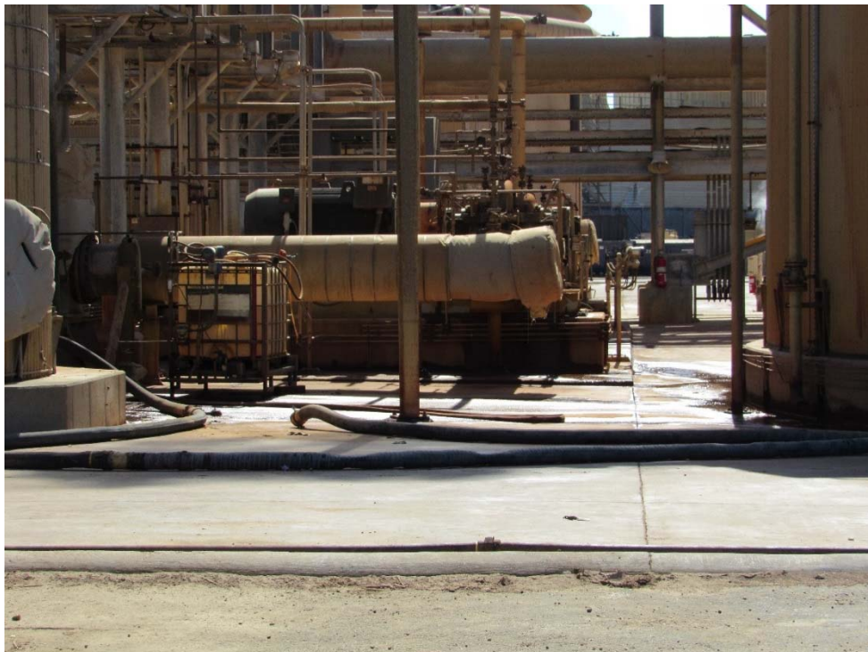
Photo 67: Looking east from the east side of the belt filter area toward the geothermal power plant.
