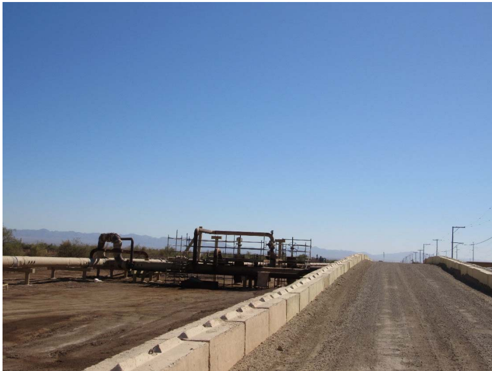
Photo 72: Looking east at the pipe crossing road that runs east and west along the north side of Mc Donald Road.
