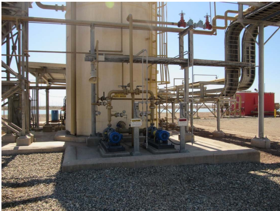
Photo 56: Looking at fresh water treatment system located at the west side of the make-up water pond.
