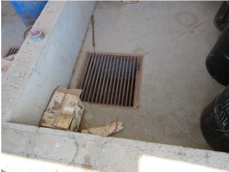
Photo 13: Looking at the sumps that are inside the secondary containment from Photo 11, these drain to the brine pond.
