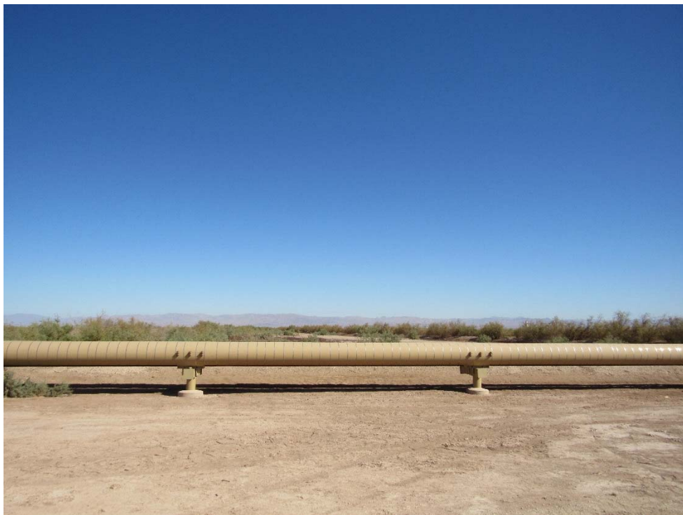
Photo 80: Looking at the geothermal pipeline that extends from the geothermal plant to the well pads.
