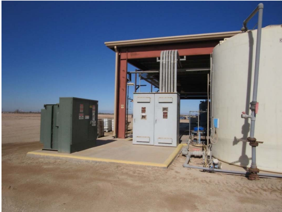
Photo 39: Looking at the southeast corner of the ES Mineral Test area at the electrical transformer and the process water tank.
