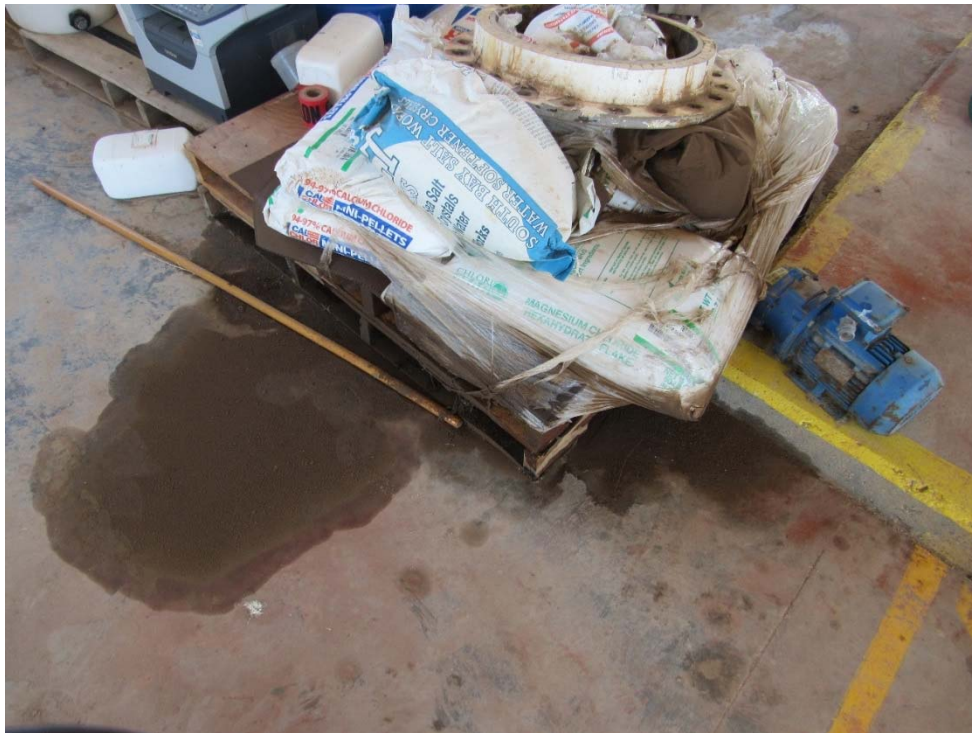
Photo 42: Looking at small hydrocarbon spill within the secondary containment at the west portion of the ES Mineral Test area of the Plant Site.
