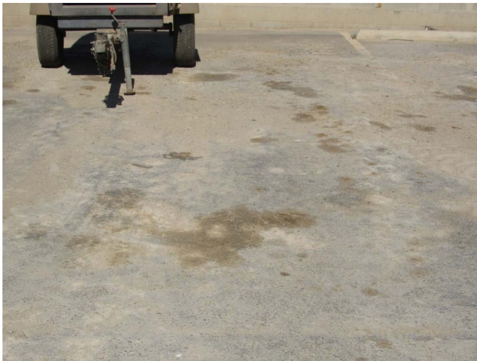
Photo 8: Looking at the slightly oil stained pavement outside of the warehouse building.
