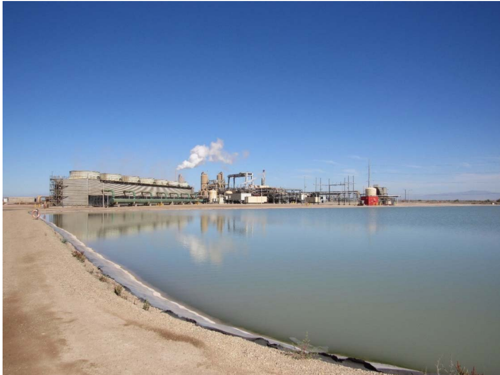
Photo 53: Looking northwest from the southeast corner of the make-up water pond toward the cooling tower and geothermal power plant.
