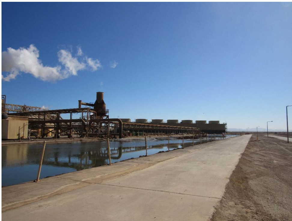
Photo 48: Looking east/northeast at the brine pond and the cooling tower in the distance within the Plant Site.
