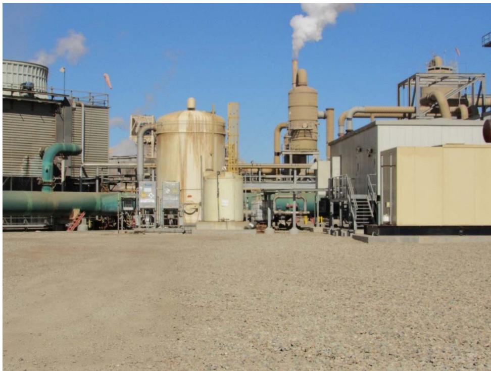
Photo 54: Looking west at the geothermal power plant from the west side of the make-up water pond.
