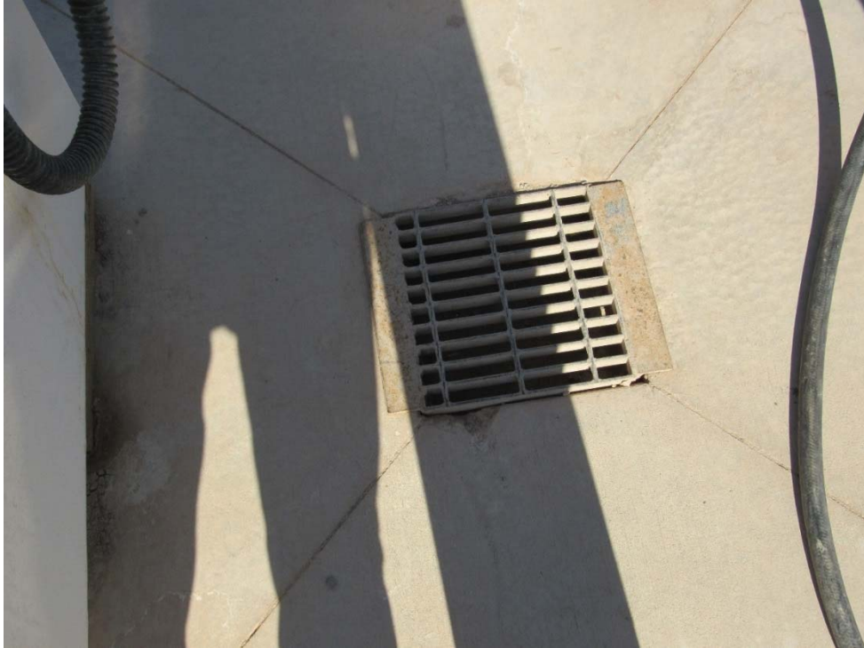
Photo 37: Looking at the drain within the fuel tank secondary containment area, this sump drains to the brine pond.
