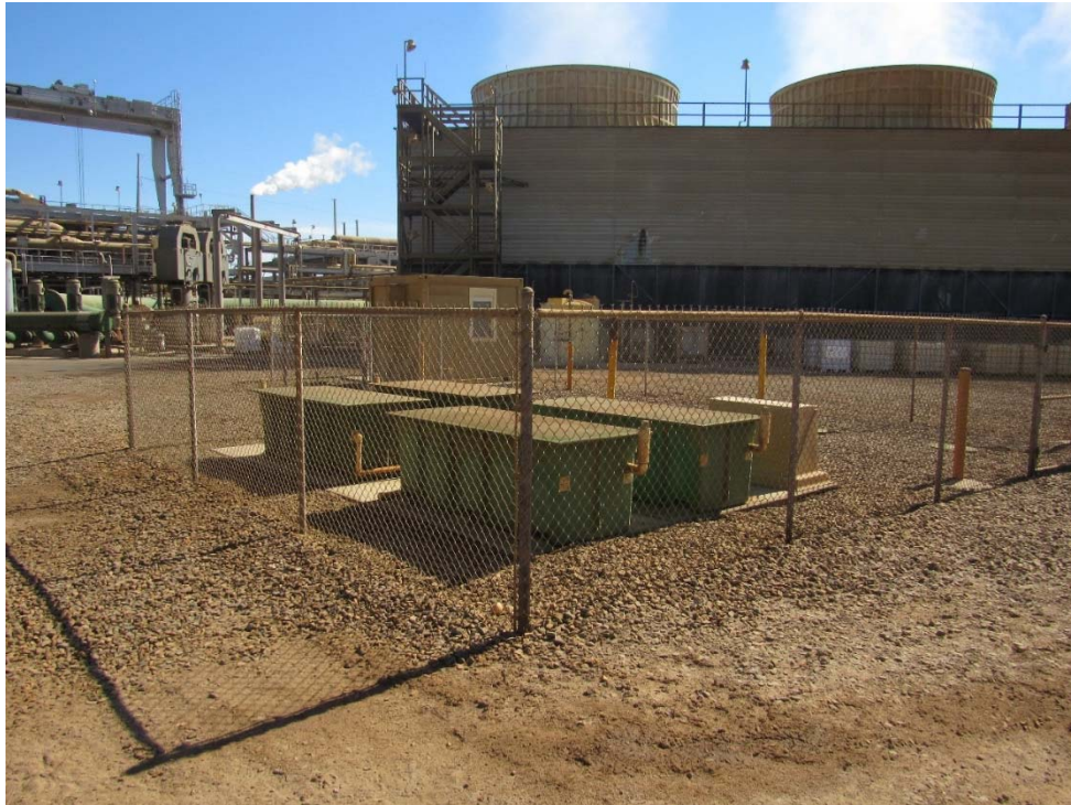
Photo 62: Looking at the waste treatment system are at the northwest corner of the cooling tower. The effluent from the waste treatment system gets reinjected with the brine into the reinjection wells.
