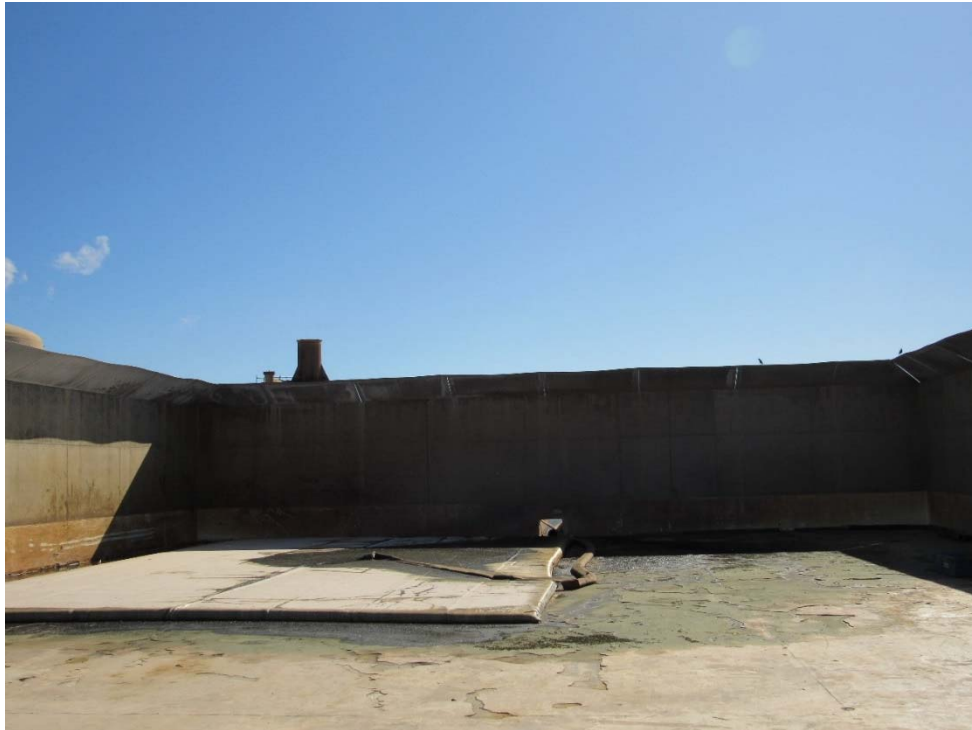
Photo 64: Looking east at the hydro blast pad, this area drains into the brine pond.
