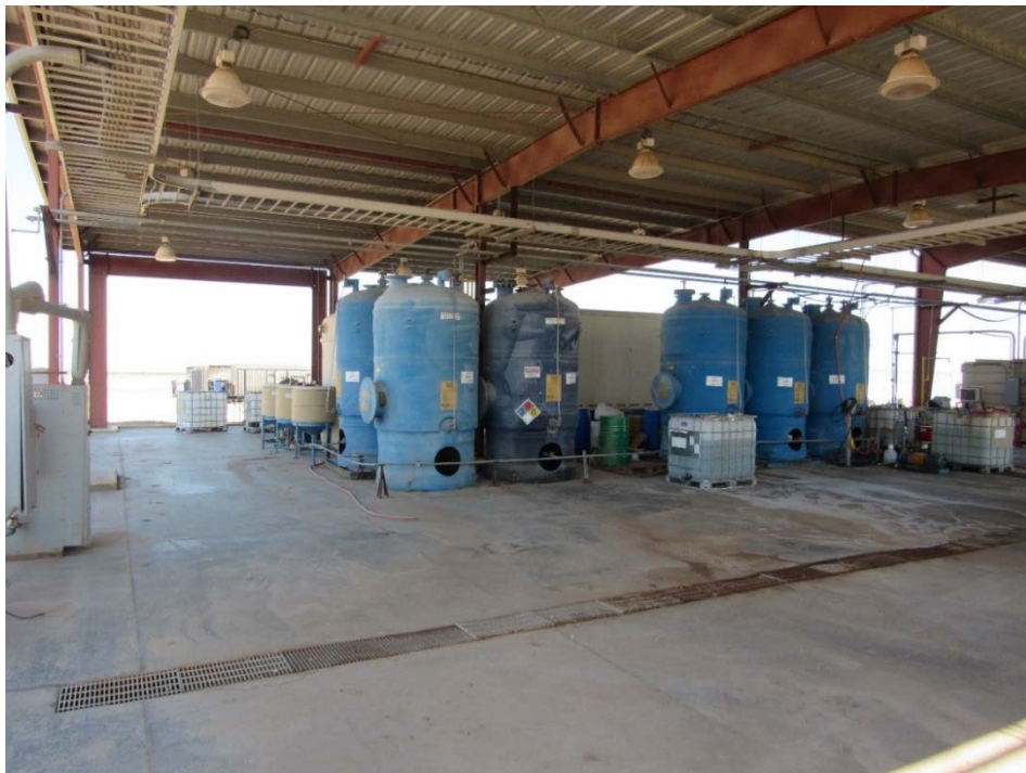
Photo 40: Looking within the southern portion of the ES Mineral Test area at various liquid containers/tanks. The blue tanks are all labeled empty. Containment curb around this area and floor drains that are connected to the brine pond.
