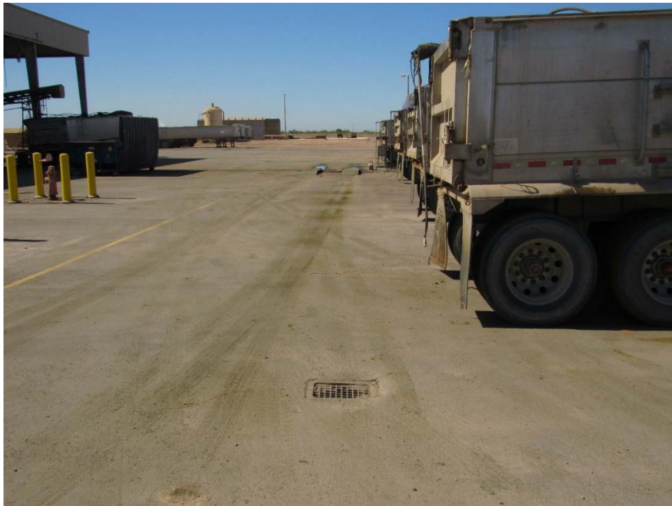
Photo 16: Looking south from the south side of the warehouse at the sumps within the paved area, the sumps drain to the brine pond.
