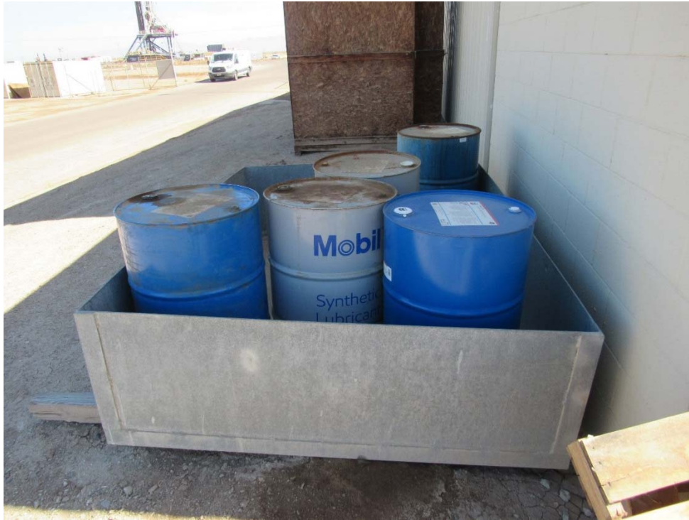
Photo 15: Looking at a temporary secondary containment bin along the west wall of the secondary containment area from Photo 11.
