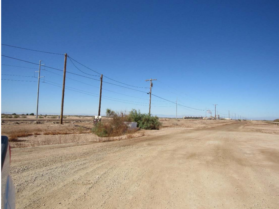
Photo 81: Looking at the Imperial Irrigation Districts pole mounted electrical transformer and water pump located at the subject property north of Mc Donald southeast corner.
