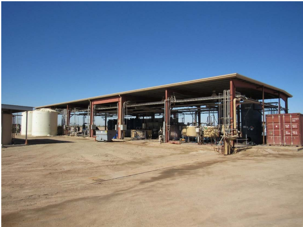
Photo 38: Looking at the ES Mineral Test area within the Plant Site, the area is bounded by concrete containment.
