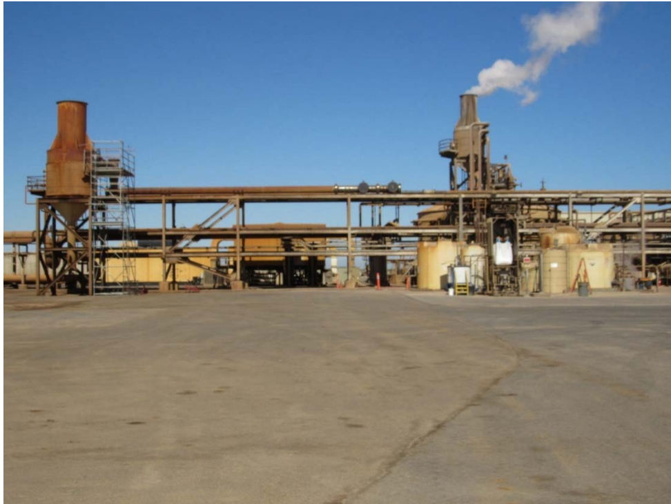
Photo 60: Looking west at the geothermal power plant from the west side of the cooling tower.
