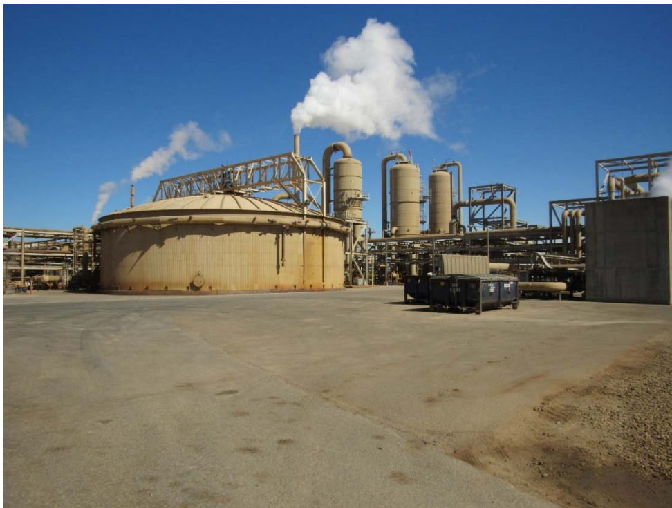
Photo 61: Looking northwest at the primary clarifier from the west side of the cooling tower.
