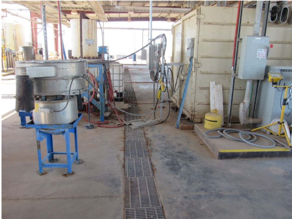
Photo 43: Looking at the drain within the ES Mineral Test area that drains into the brine pond.
