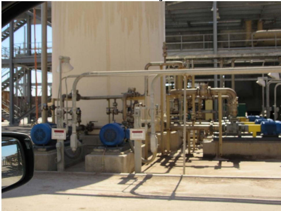
Photo 63: Looking at multiple pumps that are typical within the geothermal power plant and within a secondary containment berm.
