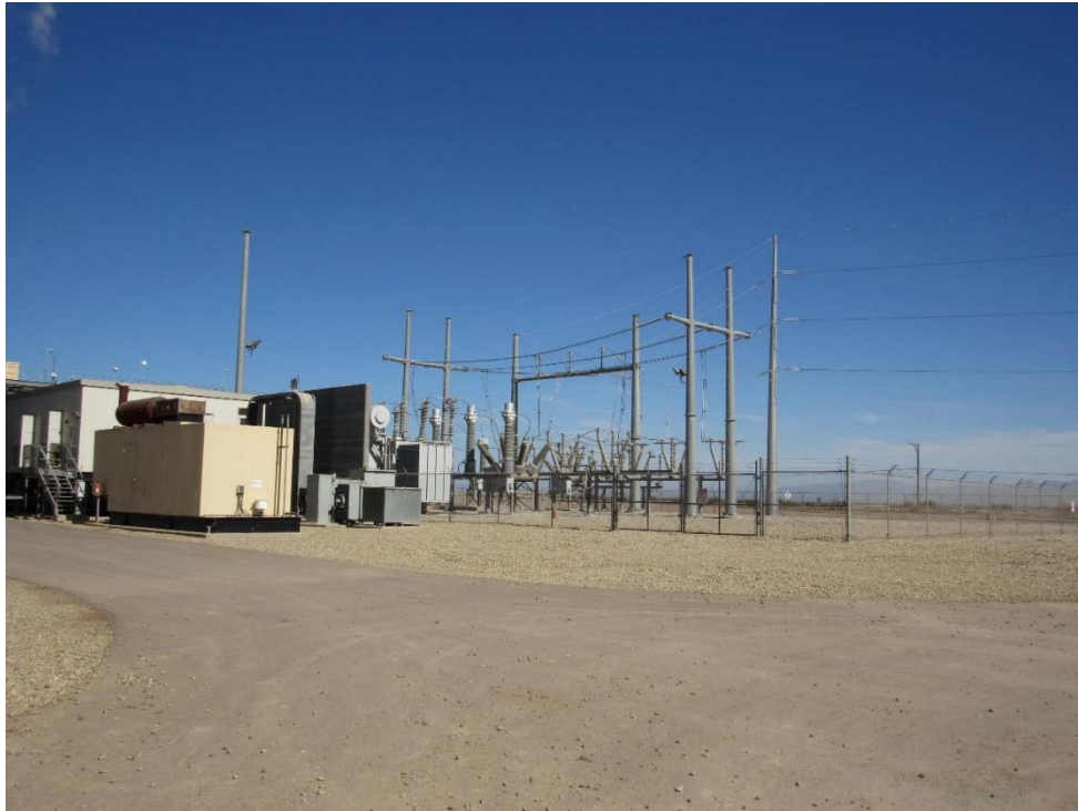
Photo 55: Looking northwest at the electrical substation located along the northern boundary of the Plant Site
