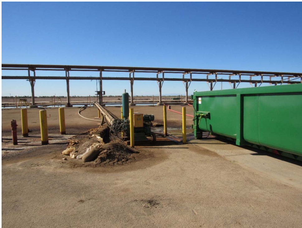
Photo 59: Looking at the sump on the north side of the brine pond. The area had recent leakage of brine during extraction into green bins, all contained and sump pumped back into brine pond.
