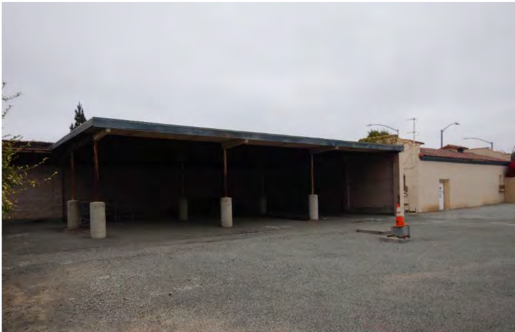
Figure 4. Carport built sometime between 1949 and 1956. The resource will be demolished as part of the project. Southern elevation of 498 Del Monte Avenue is visible to the right. View looking east-northeast.
