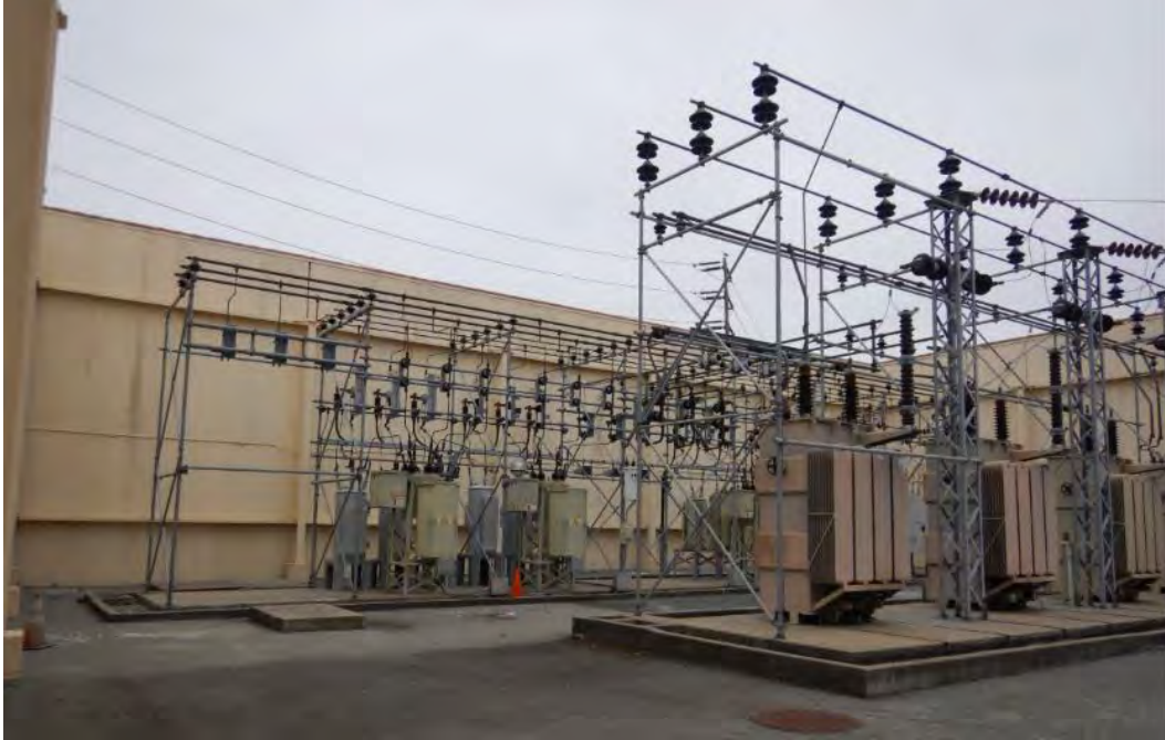
Figure 5. Substation electrical transmission equipment, installed sometime between 1962 and 1967. The tall wall that encloses the substation to the east is in the background. View looking southeast.
