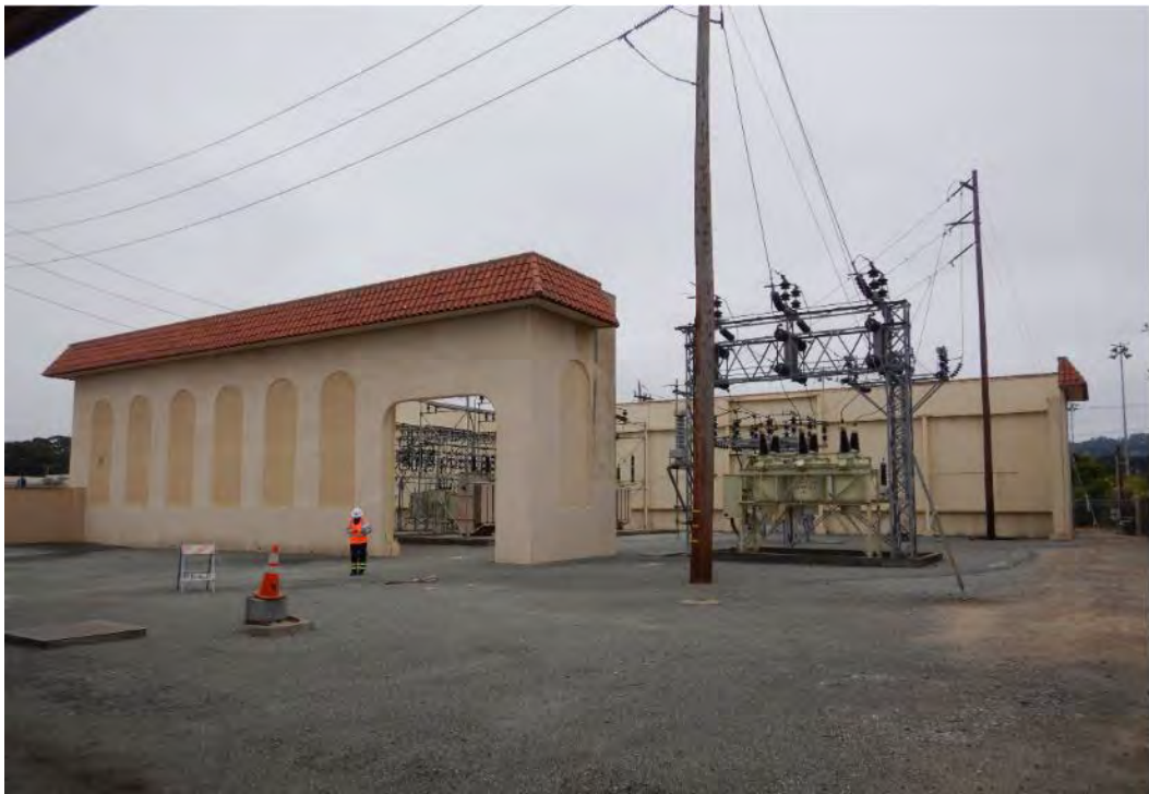
Figure 6. Photograph showing the walls that border the electrical transmission equipment to the north (at left) and south (at right). The northern wall will be removed and a new wall will be constructed or the existing wall will be relocated approximately 30 feet to the north as part of the proposed project. The northern wall will also connect to the perimeter wall. PG&E additionally proposes to widen an entrance opening in the southern wall. View looking southeast.
