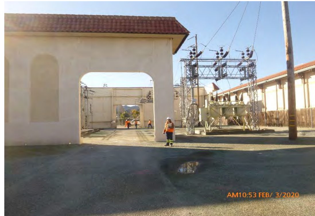
View of Project Site within perimeter walls, showing portion of excavation area (electrical equipment to be removed by PG&E), view to south
