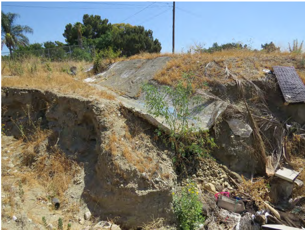
Photograph 4: Erosion at the end of the concrete lined v-ditch, and illegal dumping.
