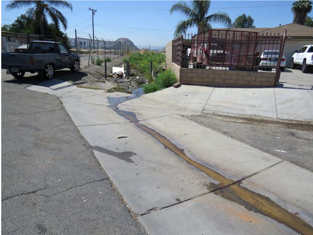
Photograph 1: Concrete lined v-ditch that is the main source of storm water that enters the northern portion of the basin.
