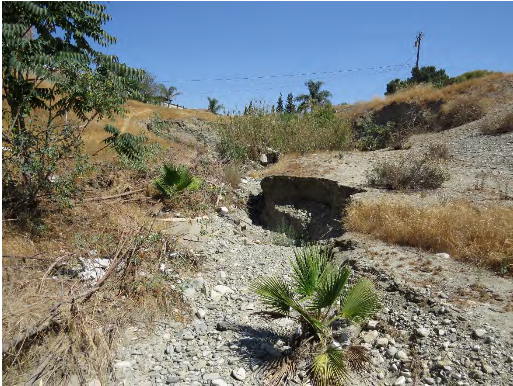
Photograph 5: Erosional area where water flows into the basin from the northern boundary.
