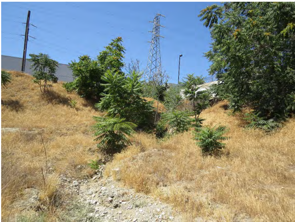
Photograph 10: Looking at the southwest corner of the basin where storm flows enter via El Rivino Road.
