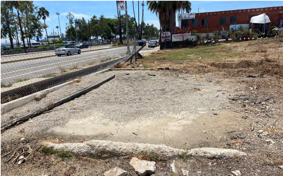
Figure 28 Concrete Foundation along Eastern Parcel Boundary of the 327 Harbor Site, Facing Southeast
