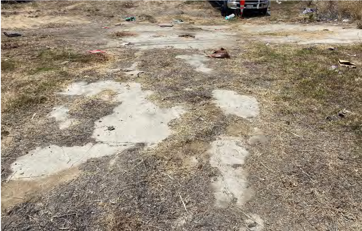
Figure 27 Concrete Foundation along Northern Parcel Boundary of the 327 Harbor Site, Plan View
