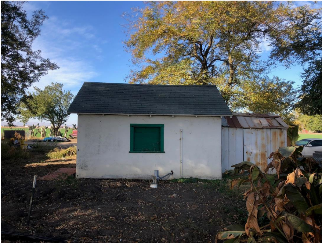
G) View of the east facing façades of the outbuilding, shed addition, looking west. 11/29/20. Acc. #MM9270
