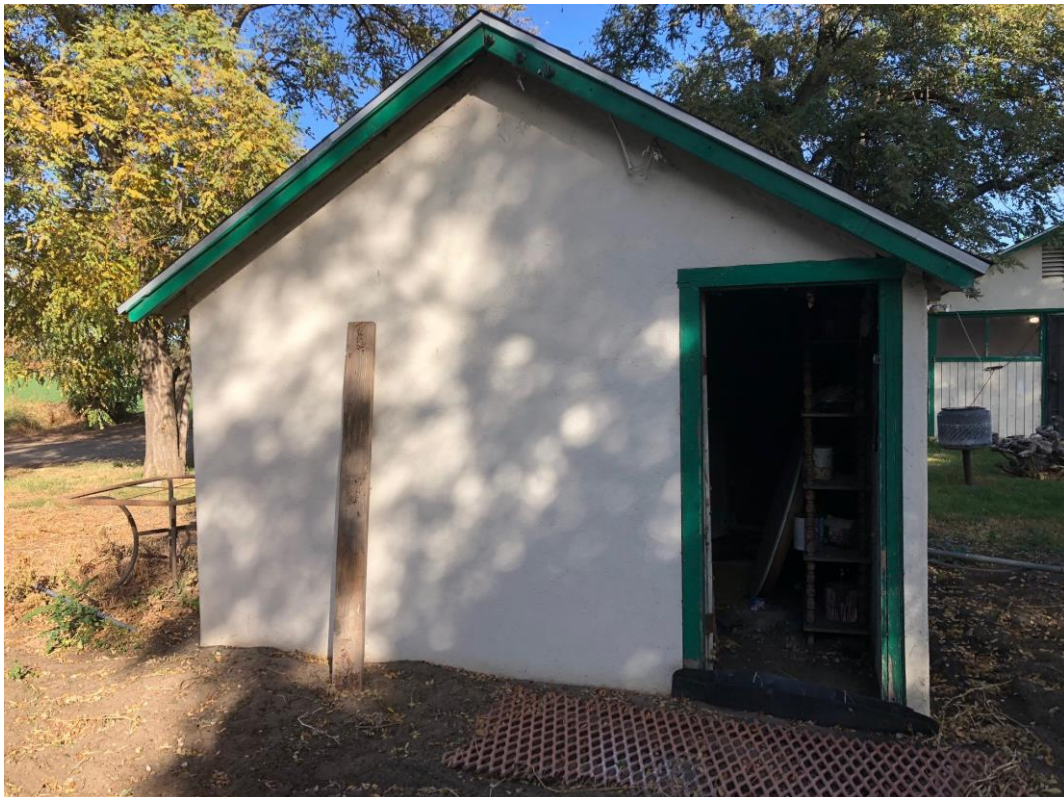
F) View of the south facing façade of the outbuilding looking north. 11/29/20. Acc. #MM9272
