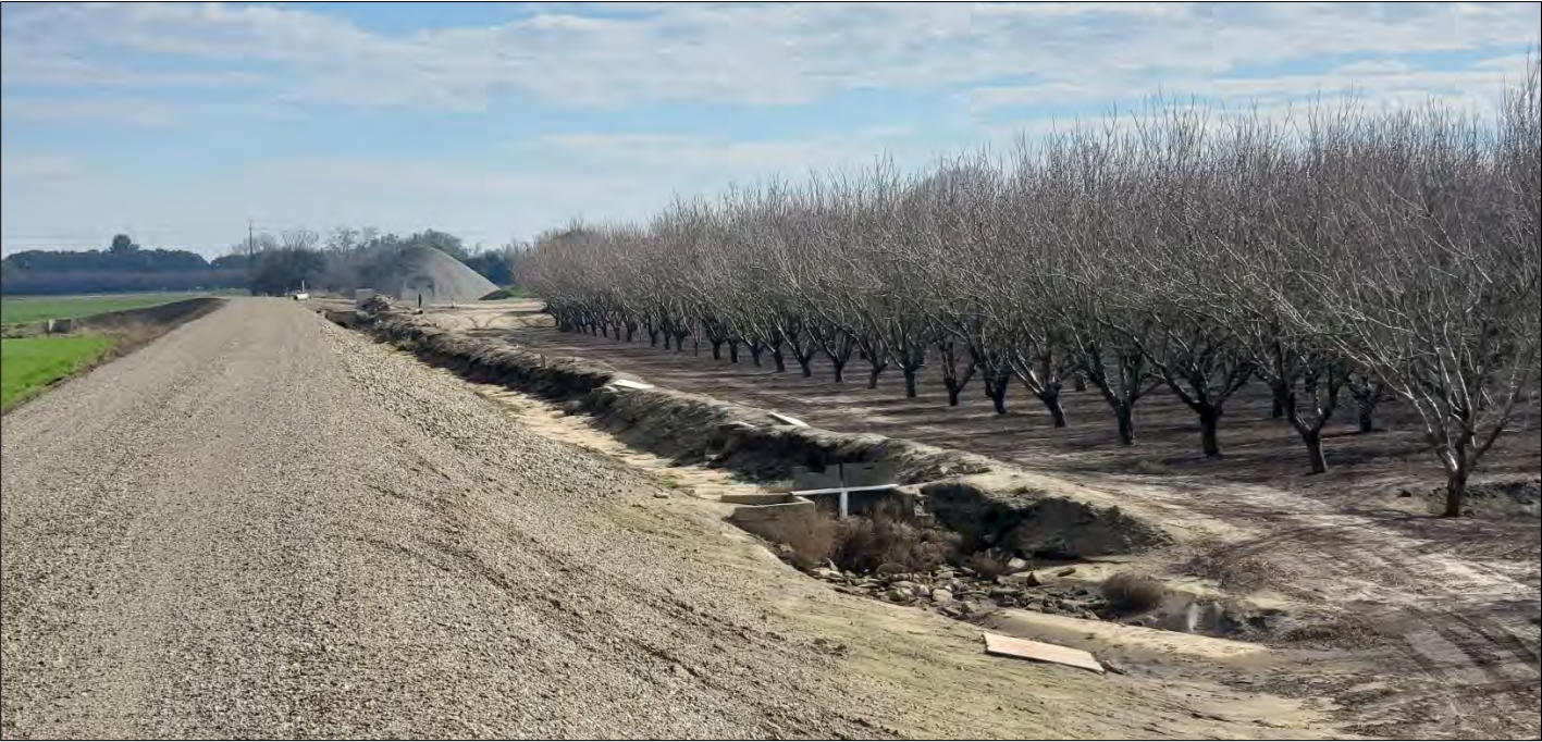
Lumina Ranch southern boundary SSJID junction box and irrigation water delivery facility photos and encroachment upon RD 17 dryland levee
