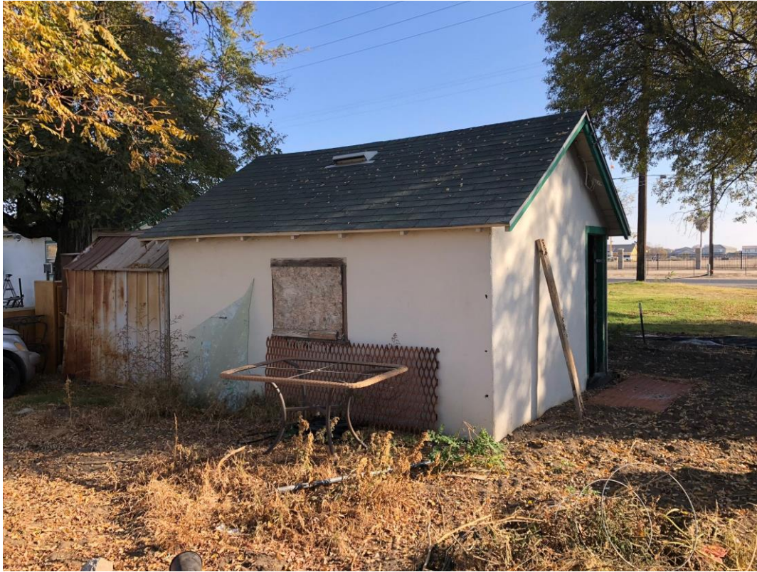
E) View of the west and south facing façades of the outbuilding looking east. 11/29/20. Acc. #MM9374
