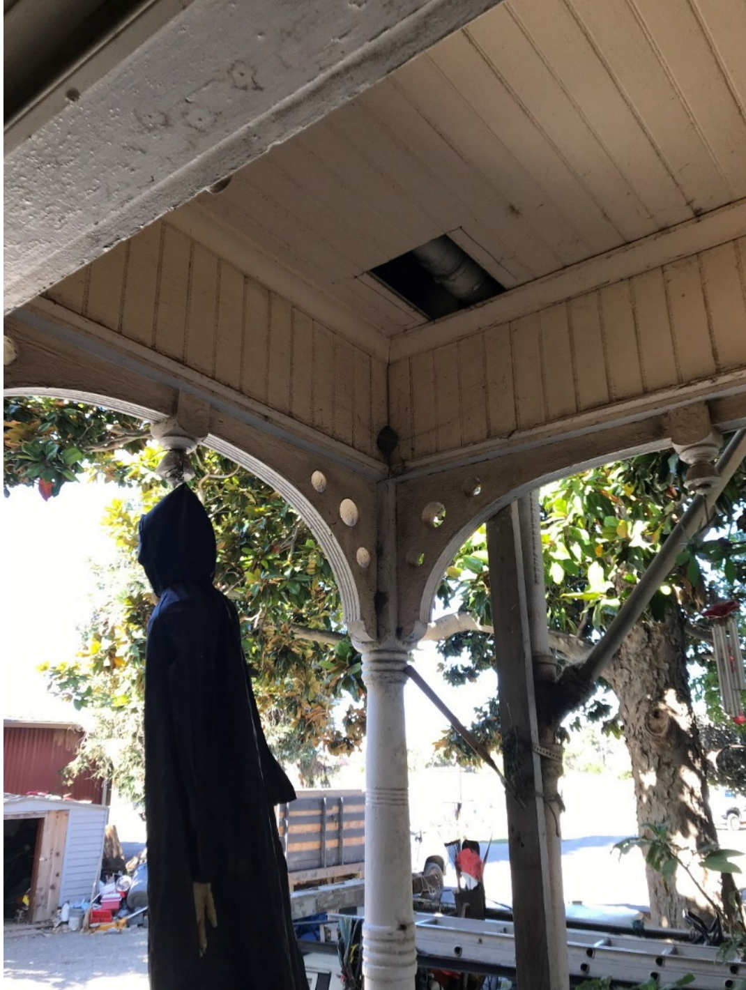
Photo 6. Facing northwest from front entrance showing probable original material construction along with minor addition; note the opening in ceiling and the vertical drain pipe.
