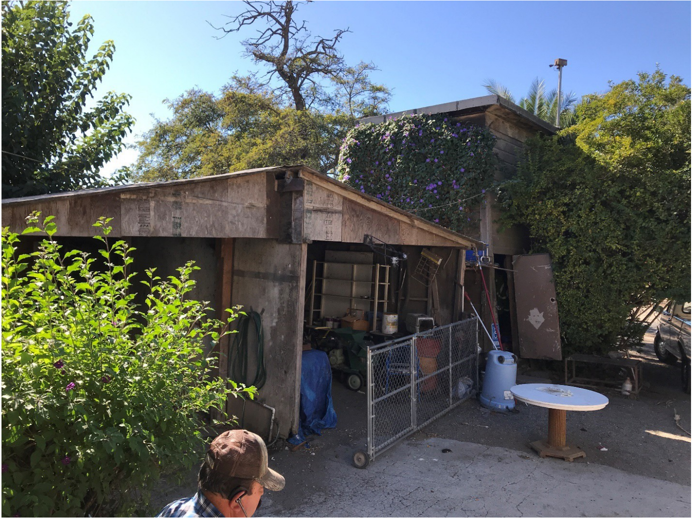
Photo 3. Facing southwest with carport in foreground and vine-covered tank house in rear.
