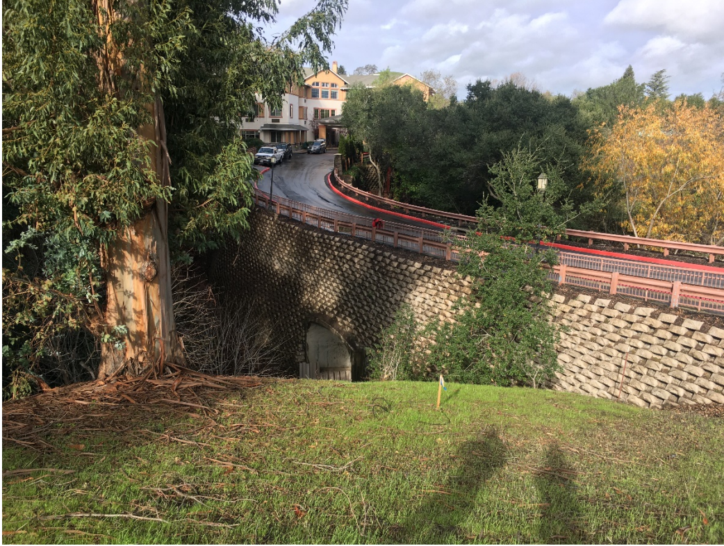
Retaining wall on east side of driveway and culvert, and assisted living facility, viewed from Pleasant Hill Road
