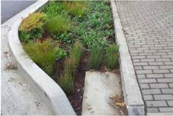
Permeable pavement sidewalk with biofiltration planter in curb extension
