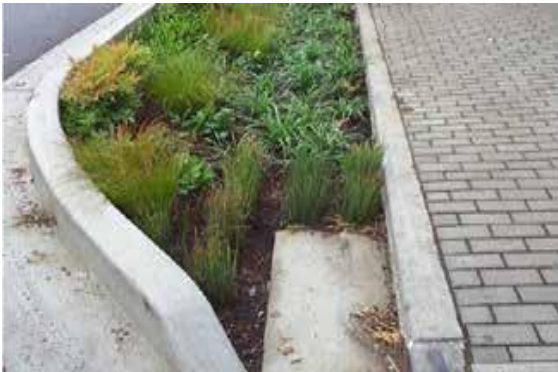
Permeable pavement sidewalk with biofiltration
