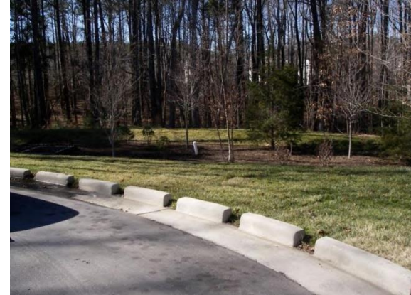
Curb cuts with filter strip
