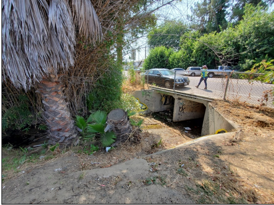
Photo 9: View of the storm drain passage under Campo Road, outside the Development Area, facing southeast.
