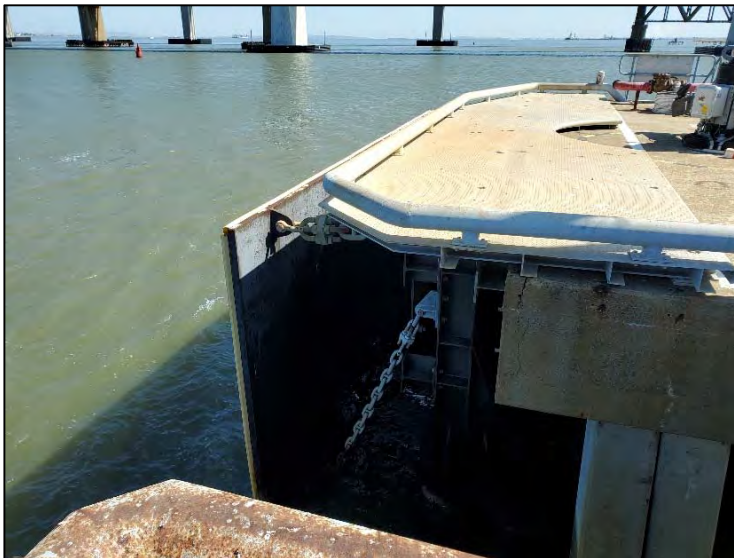
Photograph 8: Dolphin A-76 at the Amorco Marine Terminal, where concrete and piling repairs are planned.
