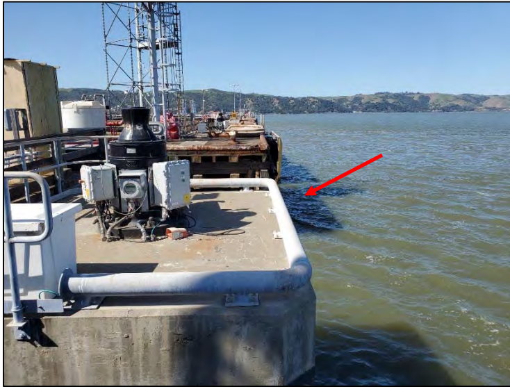
Photograph 7: Dolphin A-81 at the Amorco Marine Terminal where a new super cone fender will be mounted.
