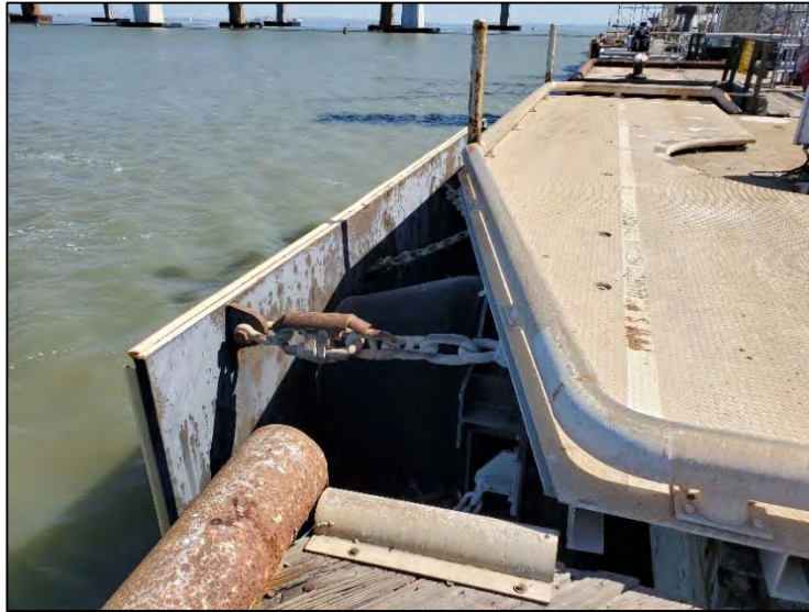
Photograph 9: Dolphin A-77 at the Amorco Marine Terminal, where concrete and piling repairs are planned, looking east.
