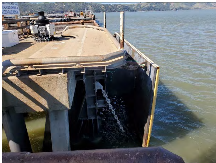
Photograph 10: Dolphin A-77 at the Amorco Marine Terminal, where concrete and piling repairs are planned, looking west.
