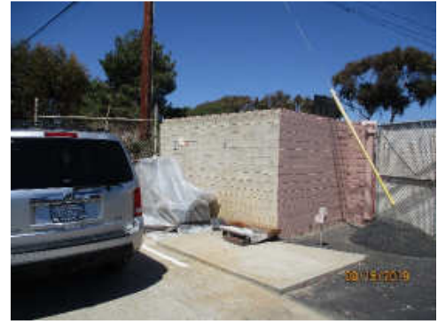
Non-hazardous waste enclosure
