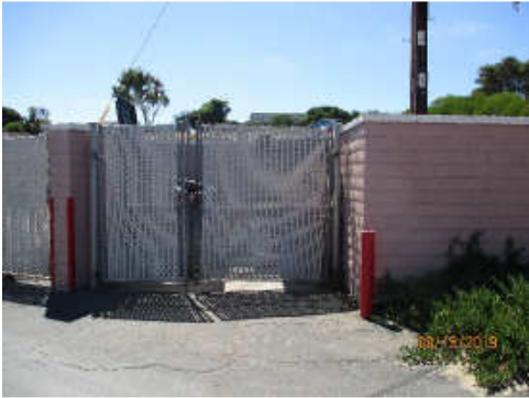
Non-hazardous waste enclosure
