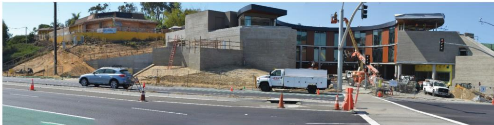
Photo 10: New hotel (Alila Marea Beach Resort) located adjacent to north of project site. Existing on-site (vacant) restaurant visible to the south.
