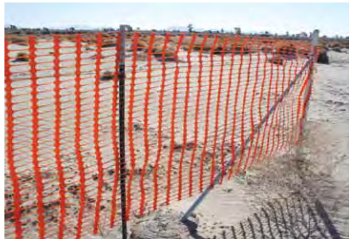
Figure 7: This 50% wind porosity fencing causes dust to deposit more on the downwind side of the fence.
