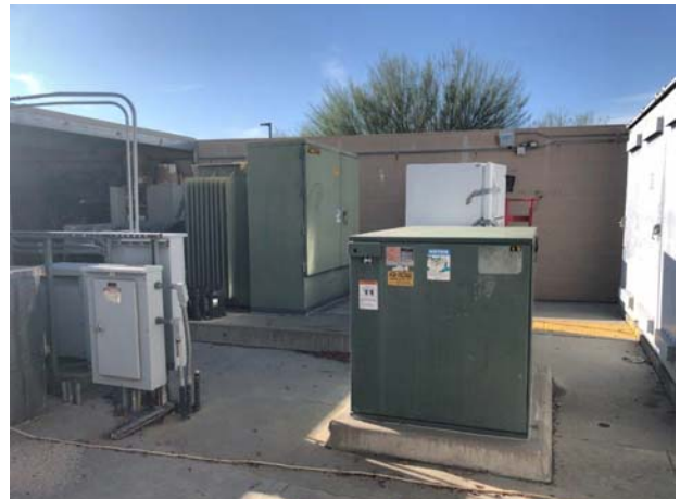
18. View of the pad-mounted transformers.
