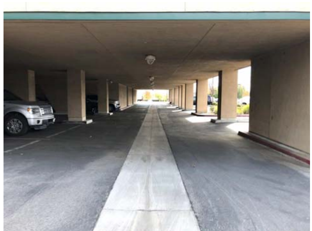
42. View of the tuck-under parking area at the west-wing of the hospital building.
