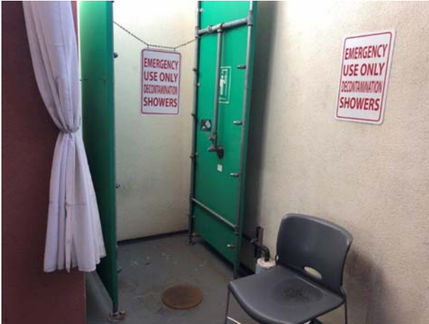
19. View of the decontamination shower and a covered floor drain.
