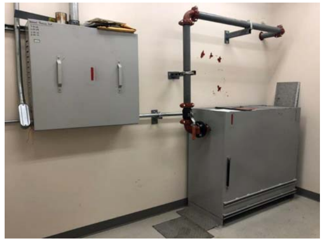
28. View of the elevator equipment.
