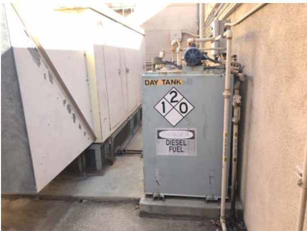
23. View of three of three emergency generators and a day tank.
