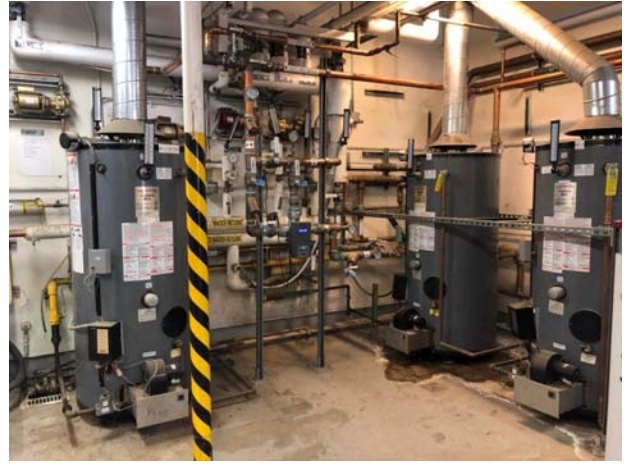
26. View of the boiler equipment.
