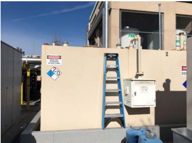
17. View of the 5,000-gallon diesel AST.
