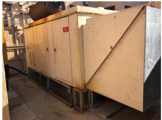
22. View off two of three emergency generators.
