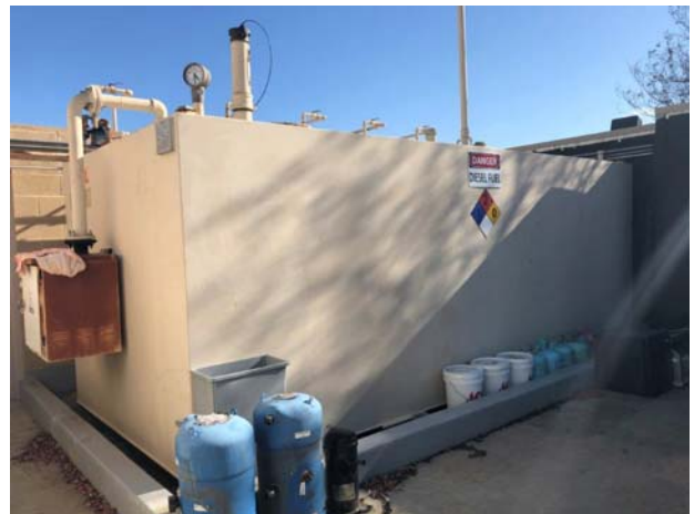
16. View of a 6,000-gallon diesel AST.
