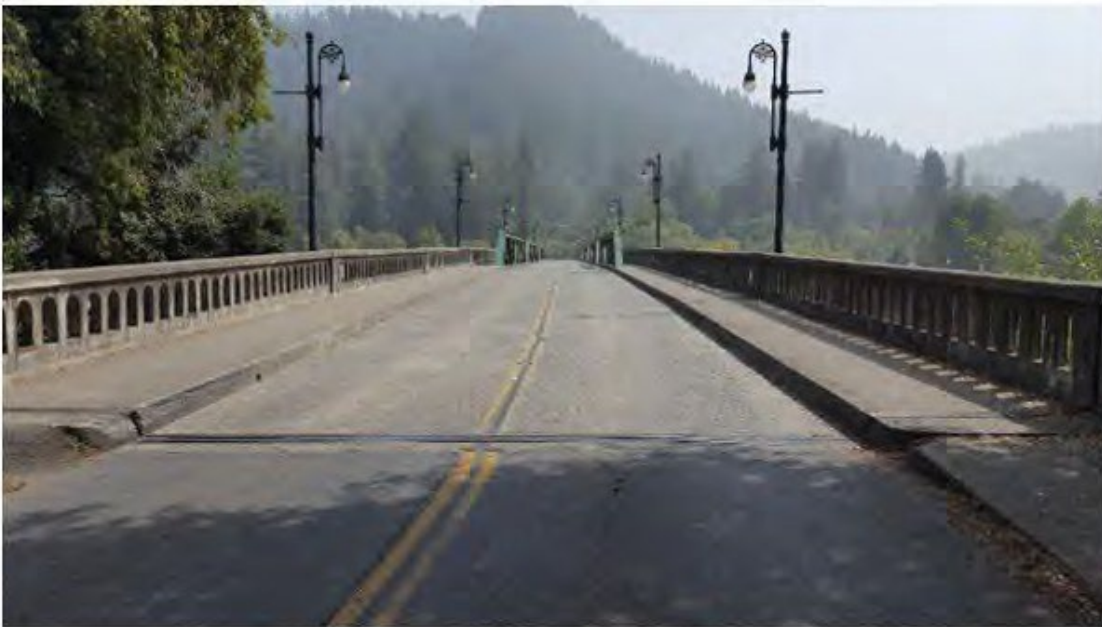
Bohemian Highway Bridge over the Russian River, looking south from the north abutment
